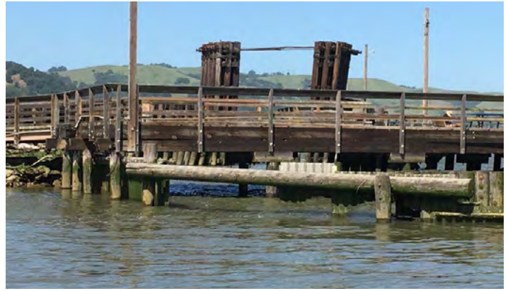
Breakwater Section A-1 – Sheet piles missing or broken
