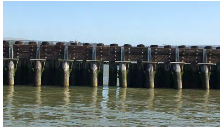
Breakwater Section B – Missing sheet pile
