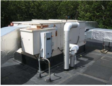
Gym Rooftop Unit
