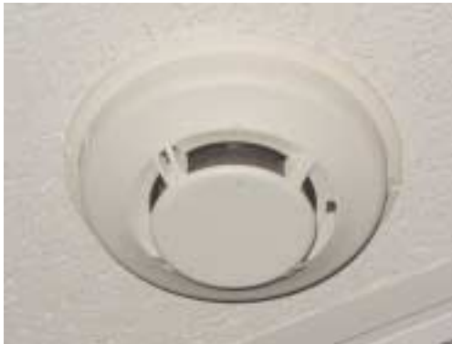
(Fig. 6.1a) Initiating device (smoke detector).
