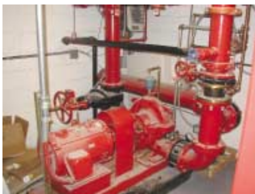
(Fig. 3.5) Fire pump.
