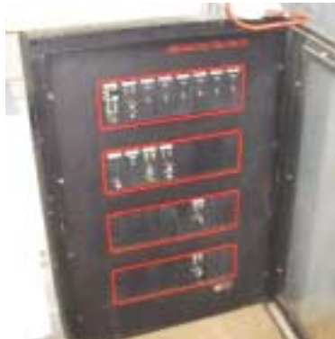
(Fig. 6.1b) Control panel.
