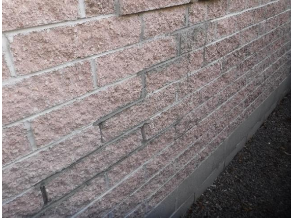
Photo 4. Moderate mortar step cracks to the Summer hill stone veneer at south east corner of the dwelling
