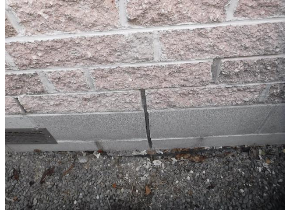
Photo 5. Moderate separation in between the concrete blocks of perimeter foundation wall.
