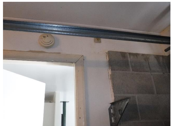
Photo 9. Minor vertical sheet separation at corner of opening to garage wall lining.
