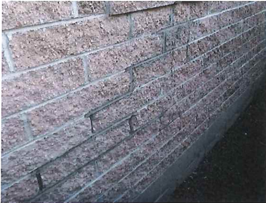
Photo 4. Moderate mortar step cracks to the Summer hill stone veneer at south east corner of the dwelling
