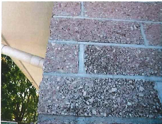
Photo 6. Minor mortar step cracks around the dwelling.
