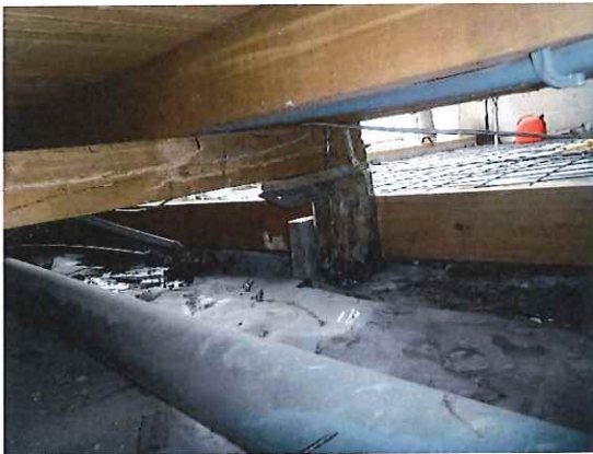
Photo 3. Single timber packer at interface of bearer and pile with steel strap connection
