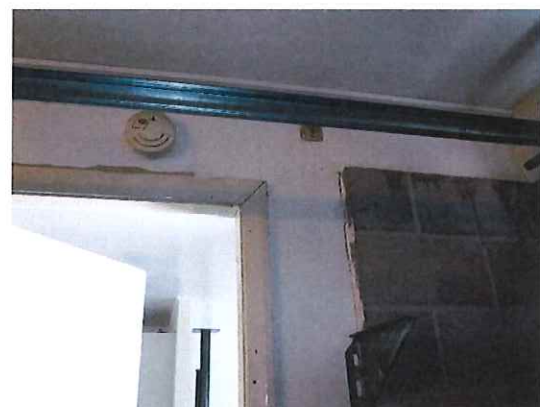
Photo 9. Minor vertical sheet separation at corner of opening to garage wall lining.
