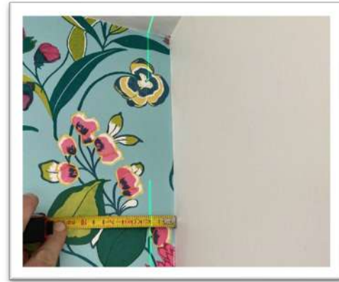
Figure 5 - Wall leans approximately 30mm over its full height
