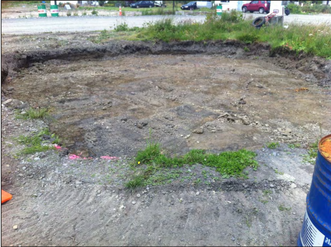
Photograph 5: View of the excavation following the removal of the impacted soils on 14 December 2013.
