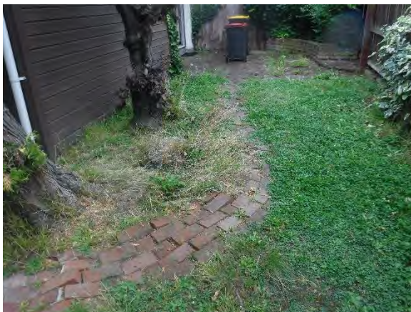
Photo 5. Undulation to the concrete pavers.
