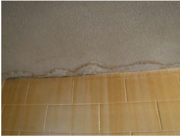
Photo 10. Water ingress identified to the unit 2.
