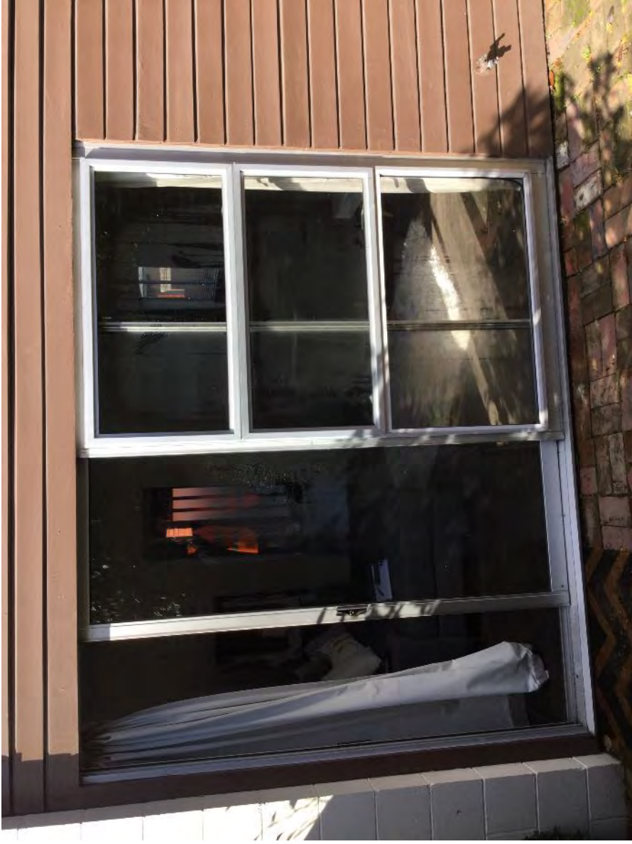
Glass slider – repaired with glass installed out of square
