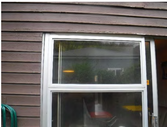
Photo 12. Door misalignment view -1 (Unit -1).
