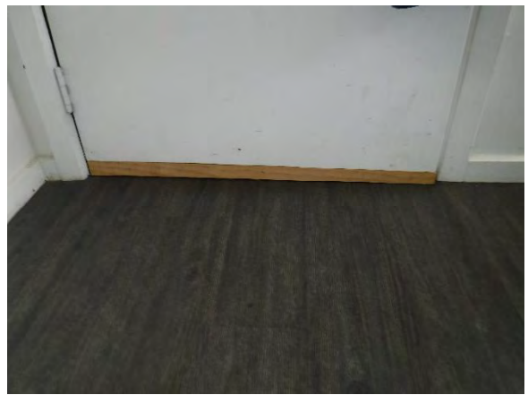
Photo 13. Door misalignment view 2 (Unit -2).
