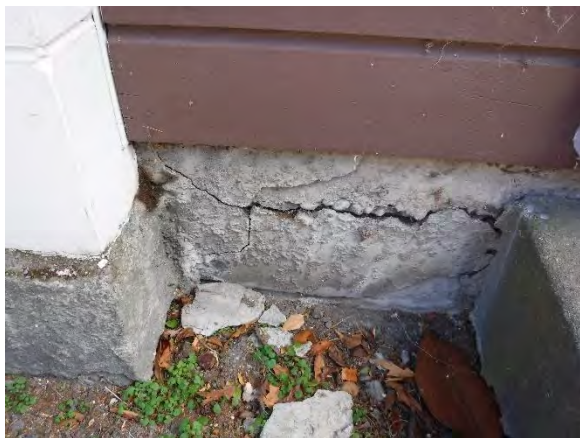
Photo 4. Cracking damage to the concrete perimeter foundation.
