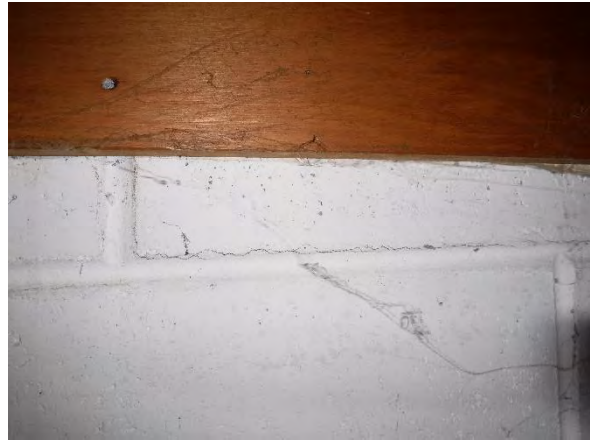
Photo 11. Minor step cracking to the block wall.
