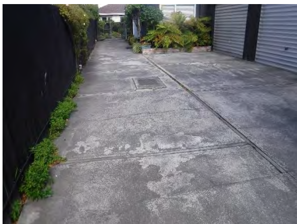
Photo 6. Cracking damage to the concrete driveway.
