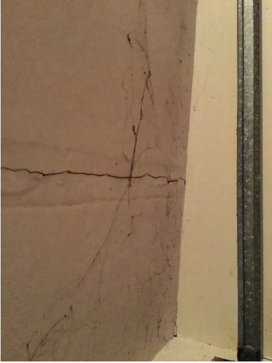
Garage- Pre Kaikoura event damage
