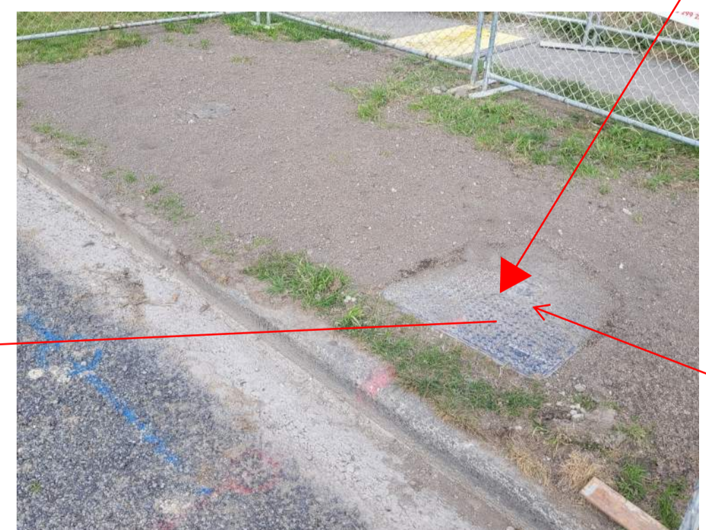
Image 2 - View under cover of recently installed Valve and vacuum point
