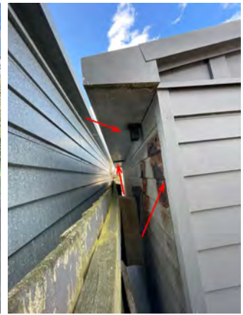
There is rusting noted on the wall cladding and the guttering and there is no down pipe, on the north face.
