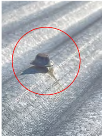
Example of raised/popped lead head nail fixings. These should be replaced with roofing screws to help with weather tightness.
