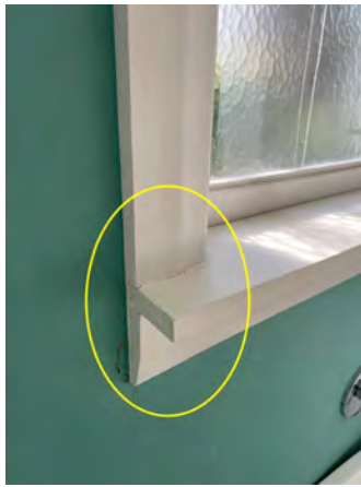
Slight signs of moisture build up here which could be contributing to the elevated moisture readings noted.
