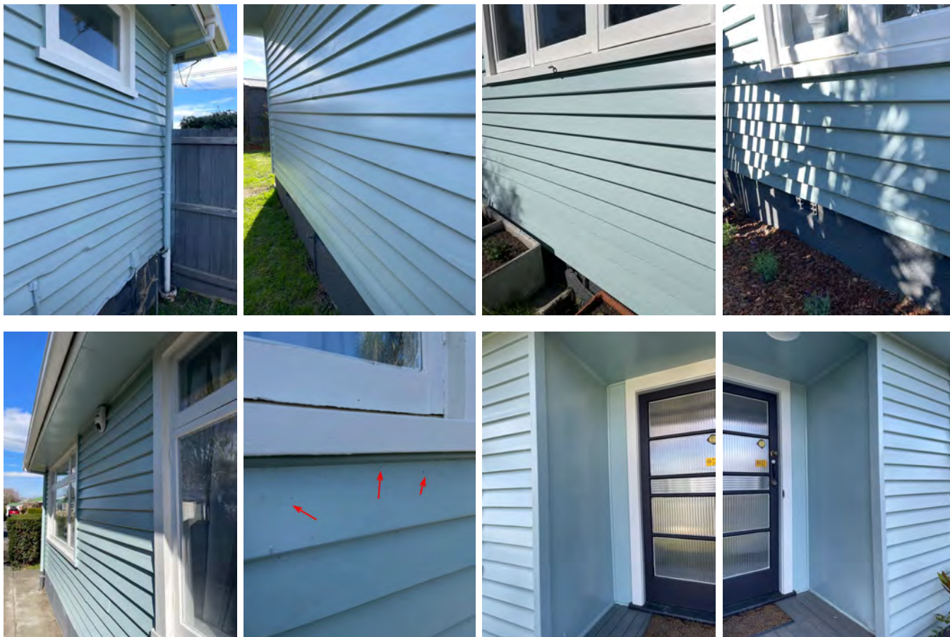
Example of signs of borer noted in the exterior cladding timber. Typical of dwelling from this age.
