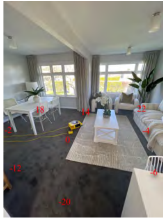
One room example of deviations in the floor heights observed during the spot level check.
