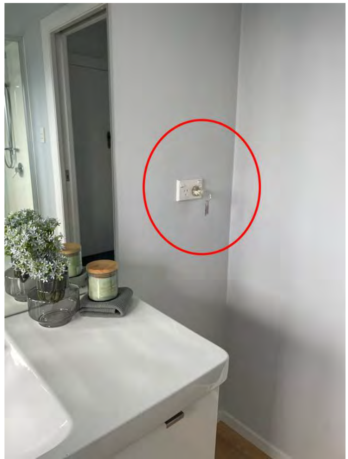
Two power sockets in the bathroom were not working.
