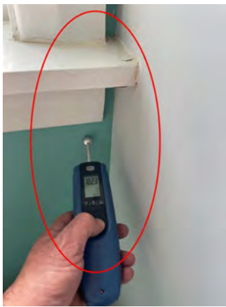
Elevated wet moisture reading in the bathroom noted.
