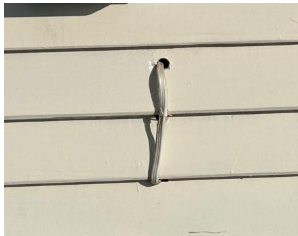
Electrical wire penetration through cladding not sealed
