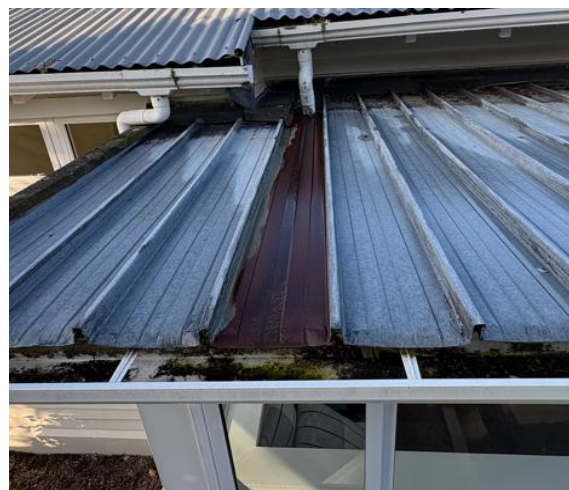
Rusted section of tray roof over entrance
