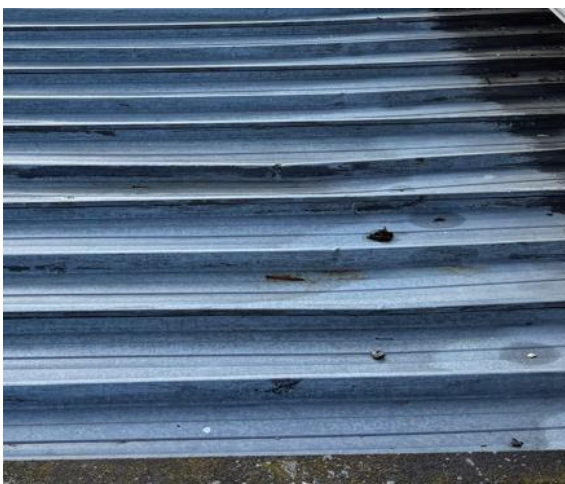
Low spot in tray roof holds water
