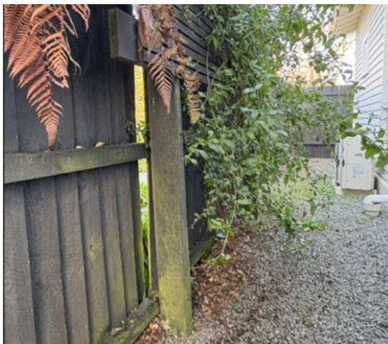
Section of fence detached
