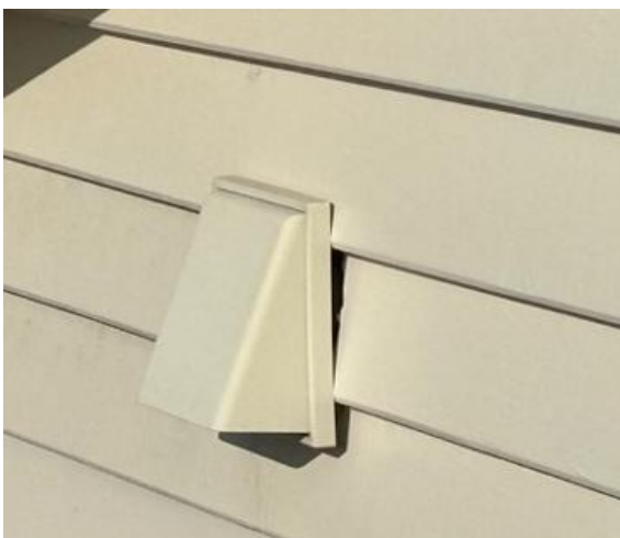
No sealant or flashings around vent penetrations
