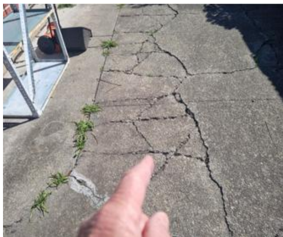
Drive – cracked and unlevel
