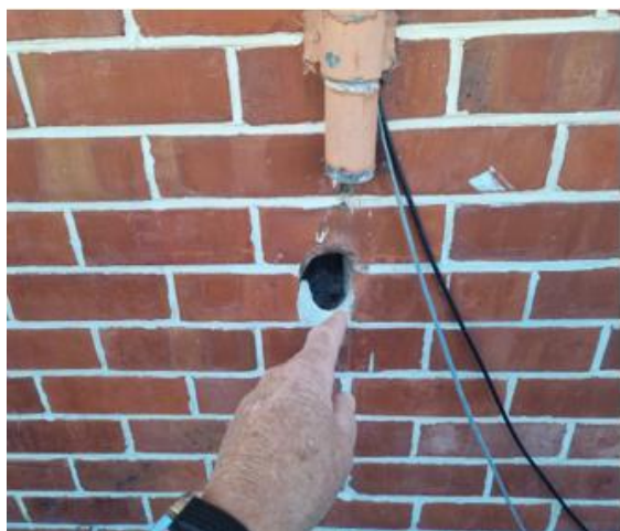
Several holes in brick work
