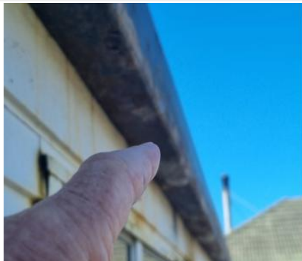
Rust to garage spouting
