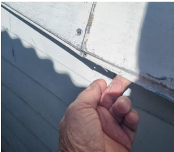
Garage wall cladding coming away from frame
