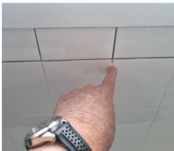
Grout missing above bath
