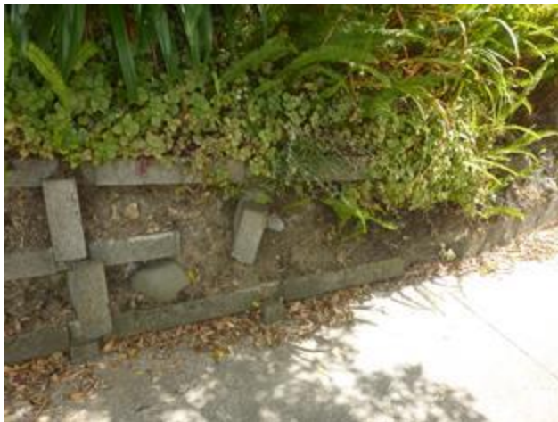
Small repair recommended
