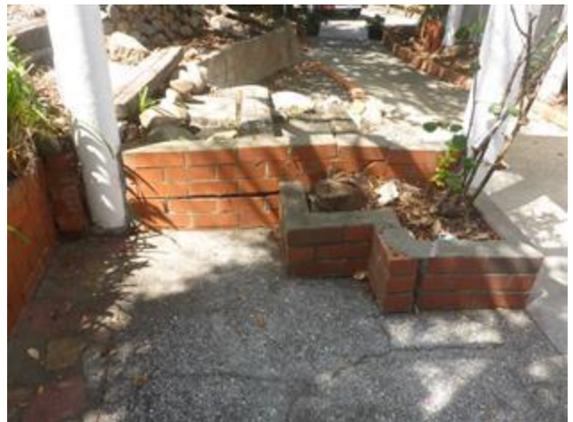
Tree root penetration
