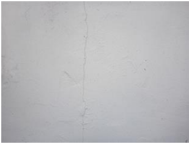
Garage cladding crack
