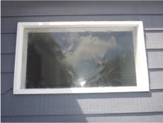
Flashing deterioration, new flashing could be retro fitted
