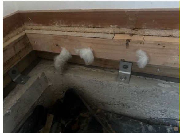
Photo 6. Over-pinning packer observed.
