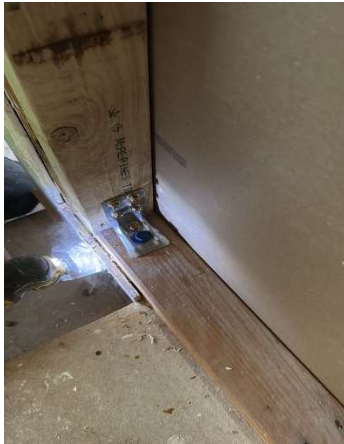
Photo 13. Hold down bracket for bracing.
