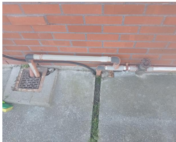
Gaps in the paving
