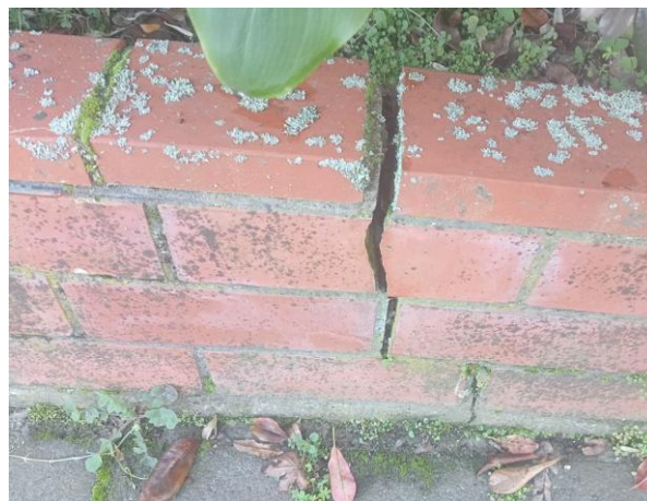
Crack in bed wall
