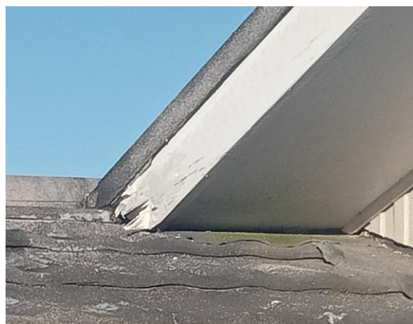
Fascia has paint peel and decay
