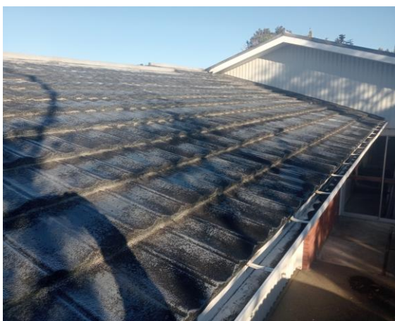
Coating loss to the roof tiles
