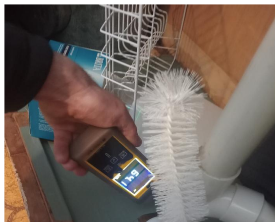
Elevated moisture readings under the kitchen sink
