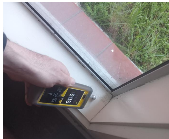
Wet moisture readings on windowsills
