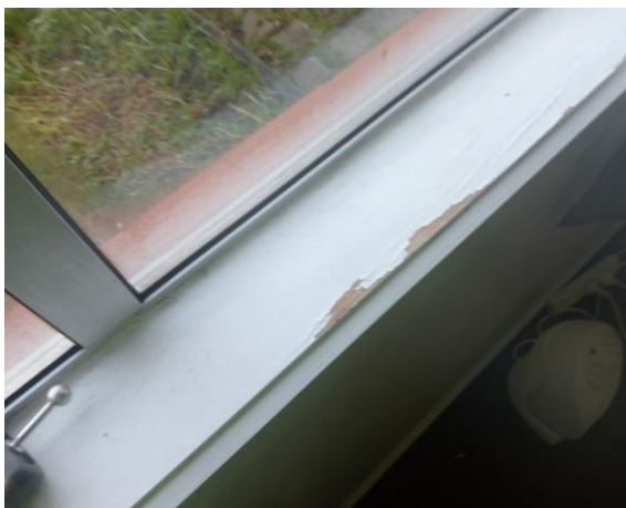
Paint peel to the windowsills
