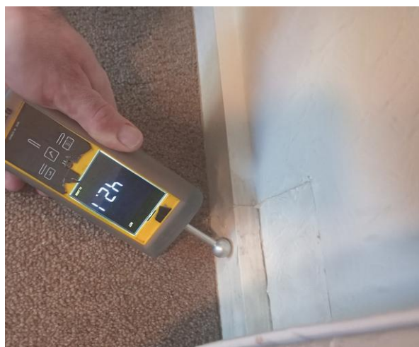
Patch on wall, join on skirting
