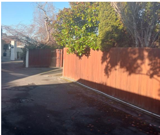
Cosmetic cracking to shared drive
