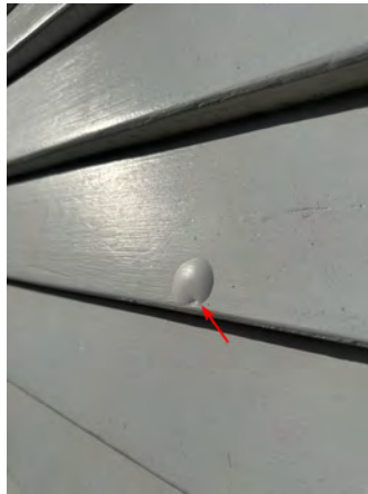
Example - paint bubbling in some spots. Strip back and touch up.
