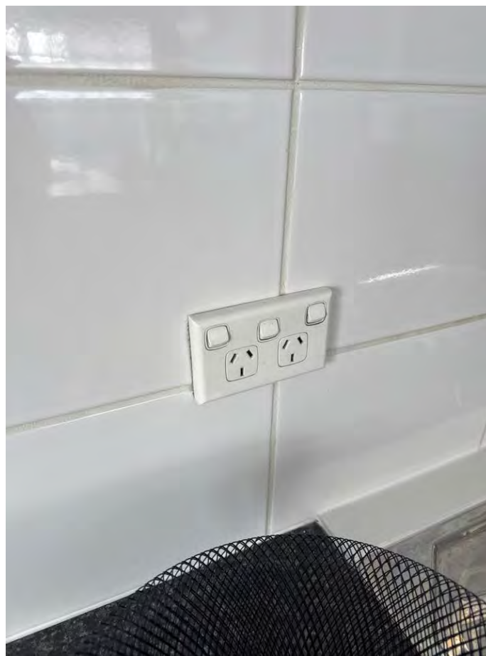
Socket is loose and needs tightening.
