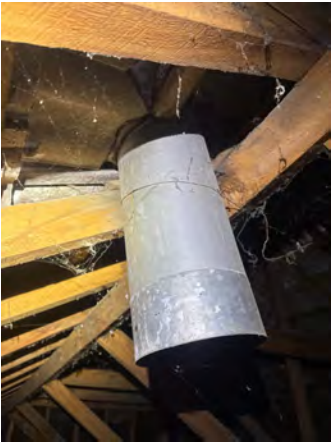
Obsolete flue could be removed.
