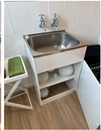
Tub cabinet is quite flimsy and should be strengthened.
