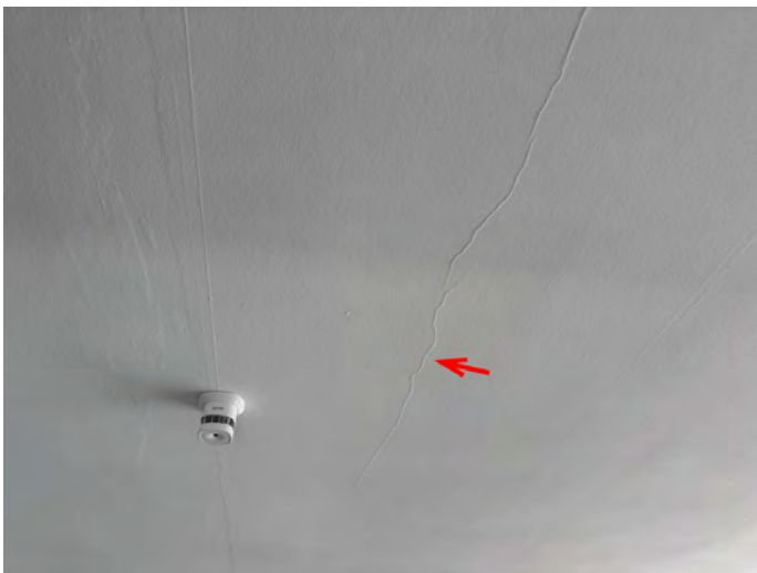
Example of cracking to lath and plaster found in many places.
