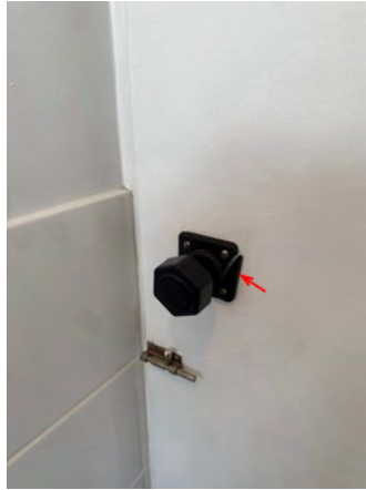
Cracked door knob in separate toilet.
