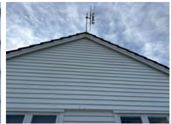
General aging and some rot under paintwork to western gable end weatherboards.
