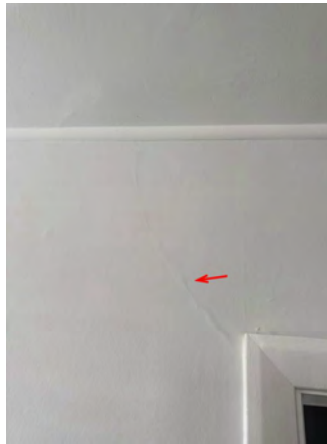
Crack under wallpaper.
