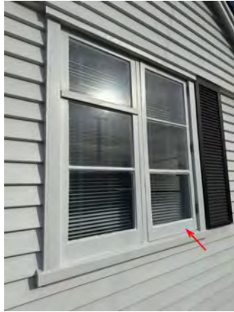
Some rot to this frame has been filled eastern elevation.
