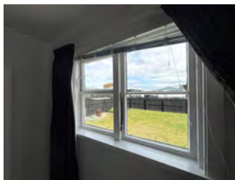
Windows are jammed.
