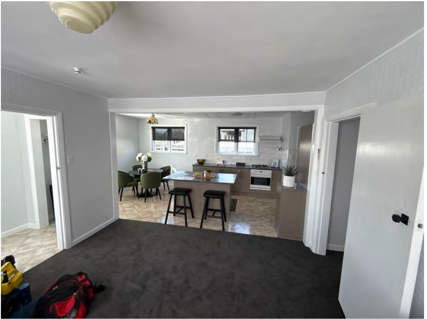
Location where load bearing wall looks to have been removed.
