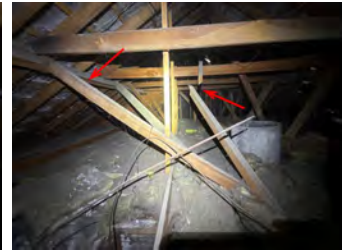
Some splitting to left diagonal brace. Reinforce this. Right side diagonal brace is broken and needs replacement.
