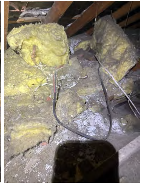
Old exposed wiring. Have an electrician check if this is obsolete.
