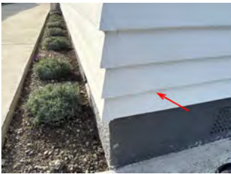
Some rot under paintwork here western corner.
