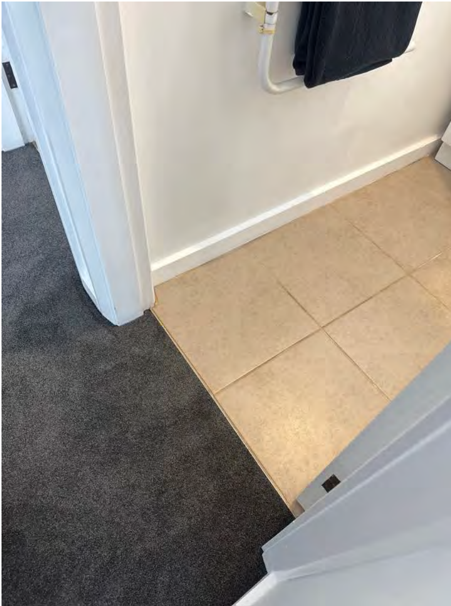
Some cracking to grout to bathroom tiles.
