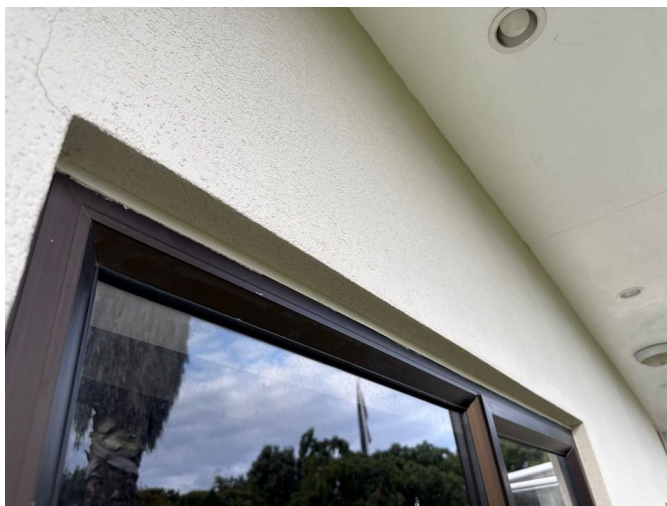
The polystyrene cladding was installed at an unknown time and was possibly installed over the original fibre cement cladding. The owner disclosed that there is no council record of this cladding addition. Note the owner has a warranty for the cladding from 2007.
