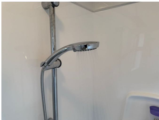
Good water pressure noted
