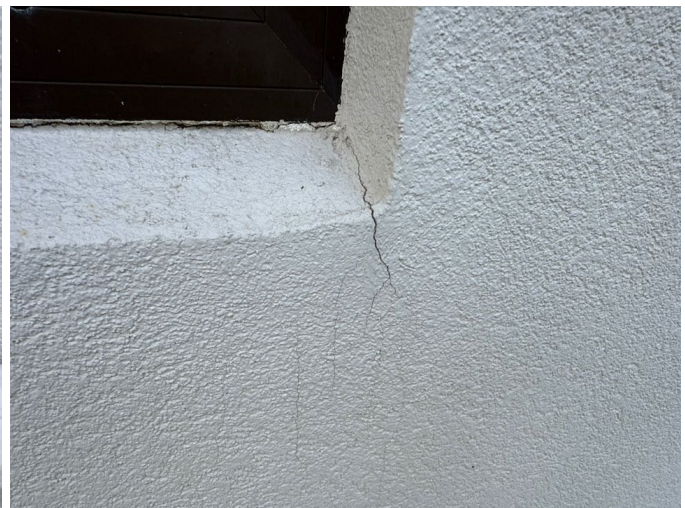
The hairline cracking is commonly the first sign that a paint upgrade is required
