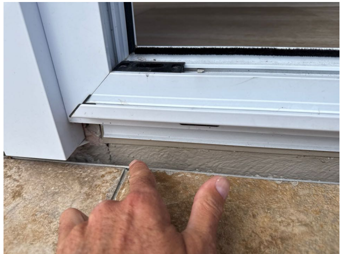
This appears to be evidence that the cladding is installed directly over the original fibre cement sheets
