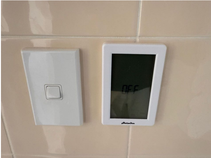
Under tile heating to the kitchen. Untested.
