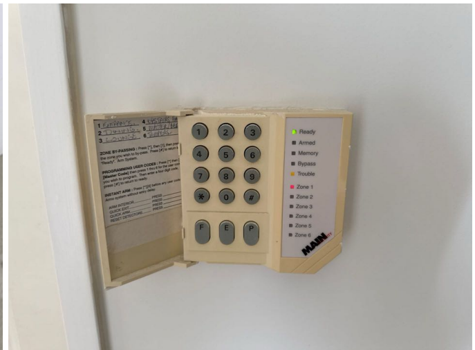
Security control panel installed by the garage
