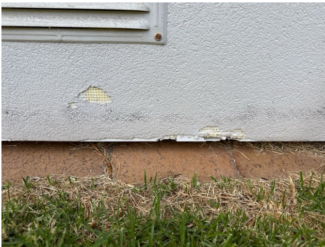
Further surface damage requires repair
