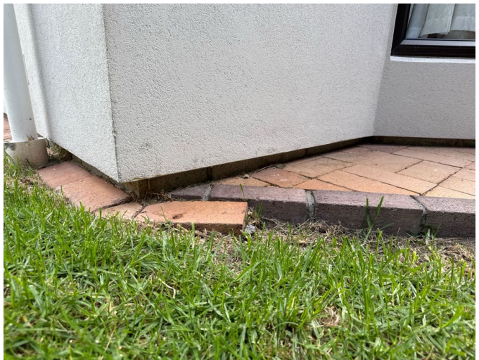
Poor ground clearance can sometimes result in moisture ingress via capillary action, a particularly high risk due to the bottom plate being at risk of decay. The current building code requires a 150mm clearance between the internal floor height and the sealed ground and 225mm to unsealed ground. At the time of the inspection all non invasive moisture tests completed to the bottom plate at these locations presented within the acceptable range.
