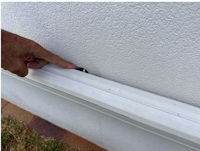
This hole in the cladding is a high weather tightness risk. Water proofing improvements are required.
