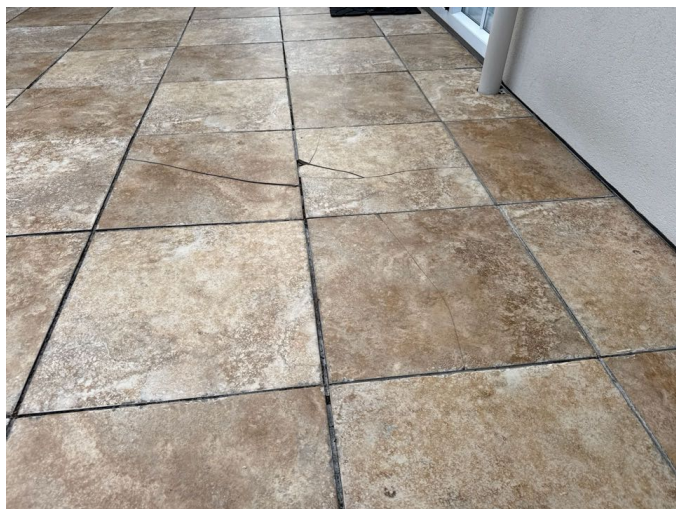
Damaged tiles to the north side should ideally be replaced
