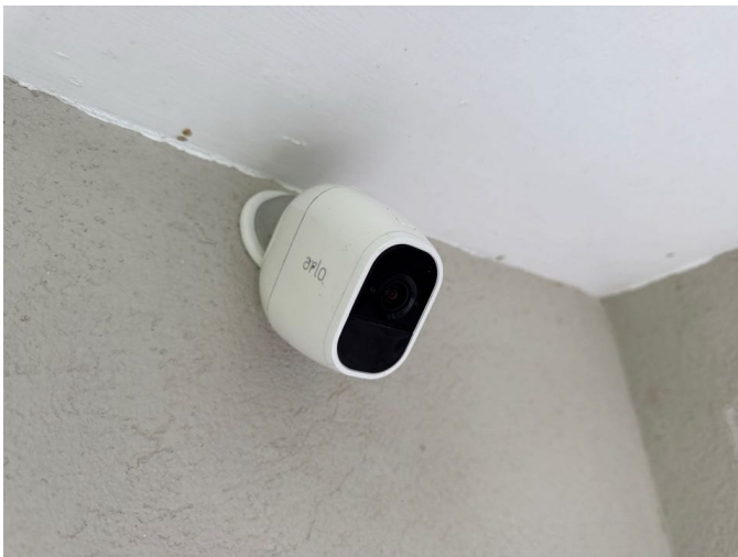
Security camera system installed. Untested.
