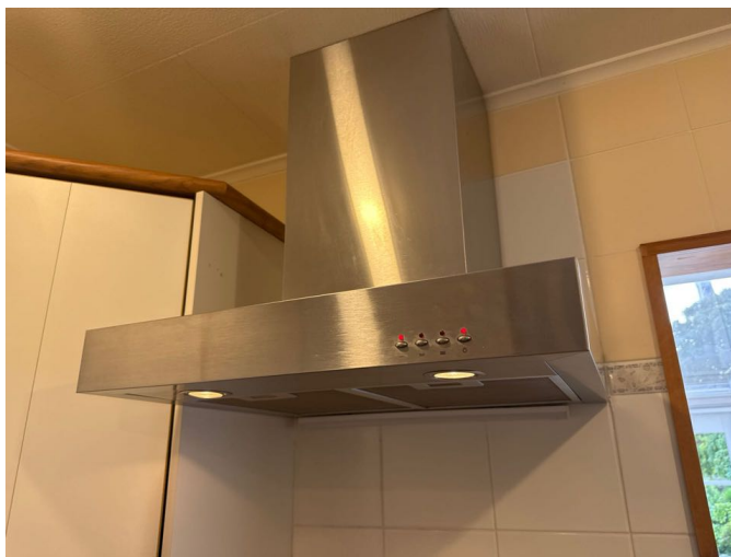
The range hood extraction unit is functioning
