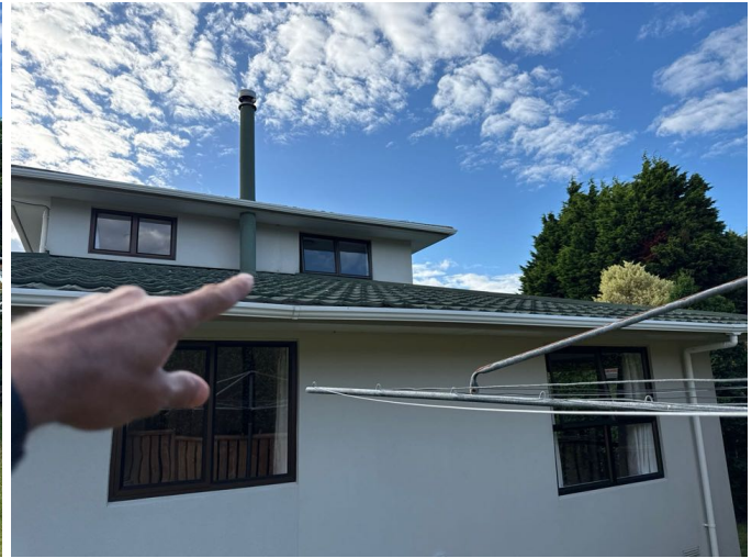
Damage to the cladding requires professional repair
