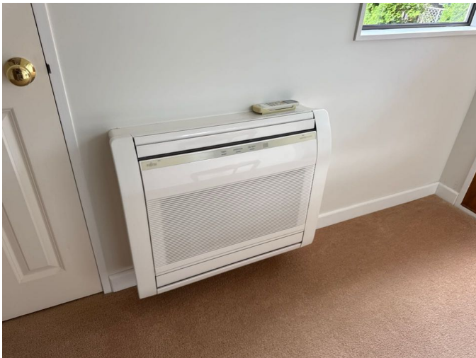
Heatpump to the east end of the hallway by the entrance. Untested.
