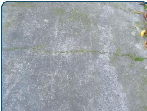
example of cracking to paths appears sound.
