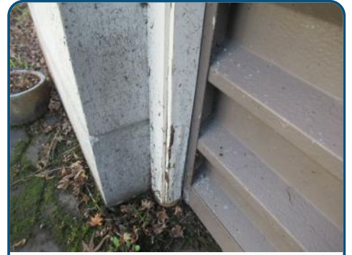
example of soft timber trim on garage at small door noted.
