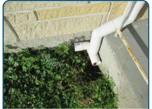
example of downpipe needing directed to appropriate outlet noted.
