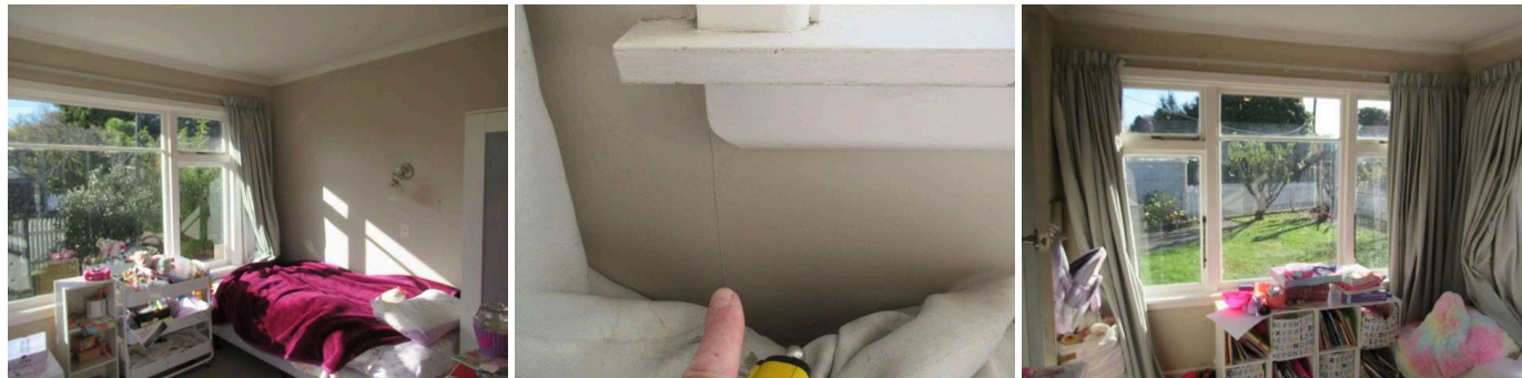
sheet joint movement noted
