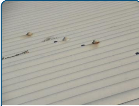
example of surface rust to roof fixings noted
