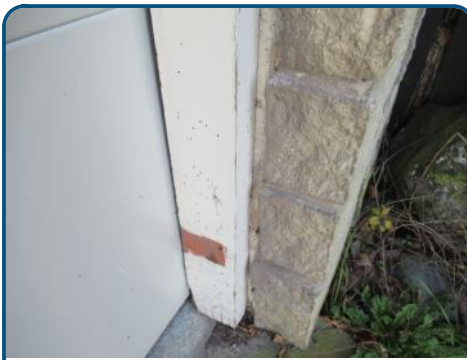
example of borer holes in garage timber trims noted
