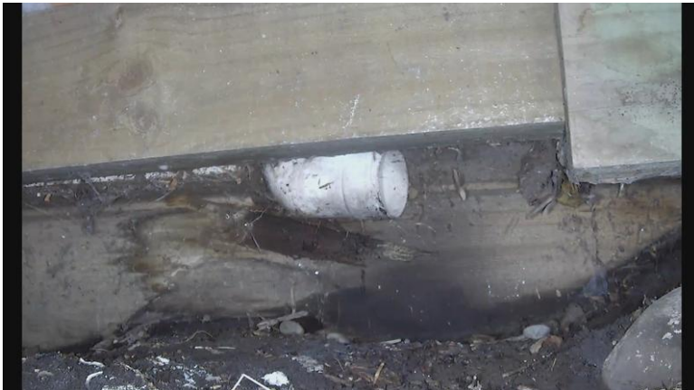
Photo 65 South side downpipe discharges under the house.
