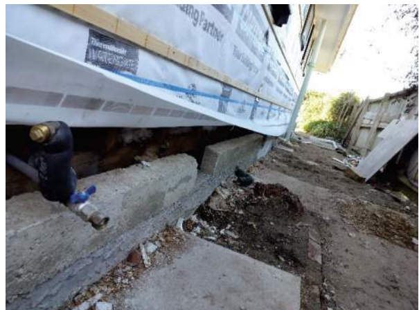
Photo 6. View of the partially replaced foundation.
