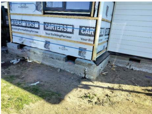
Photo 5. View of the repaired crack on the perimeter foundation (1).
