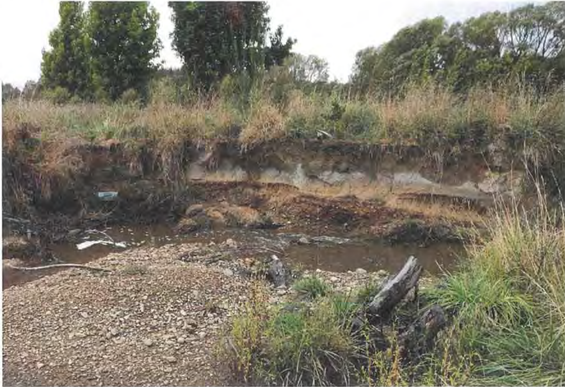
Figure 6: Bank exposure at Stringer Creek below box culvert and adjacent proposed Lot 2
