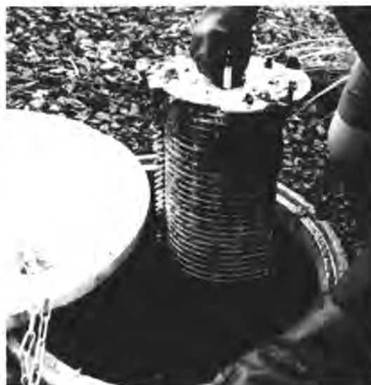
Figure 14: Servicing of a Lifestyle system is completed every 6 months
