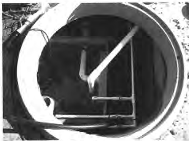
Figure 6: Pump out chamber
