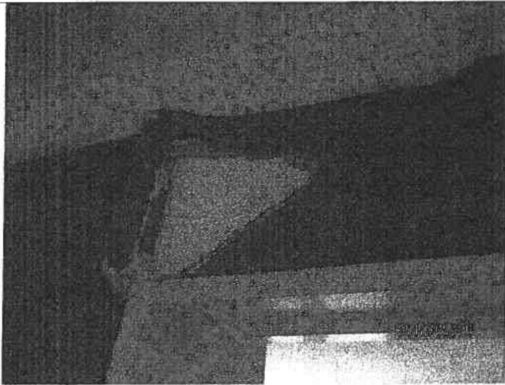
Significant Gib wall crushing above door in entry
