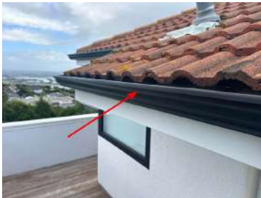
Colour steel gutter system
