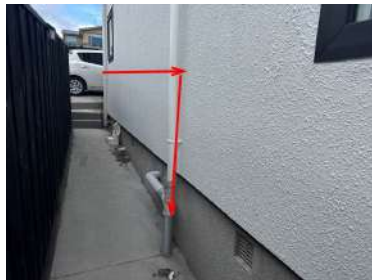
All downpipes directed into stormwater as intended
