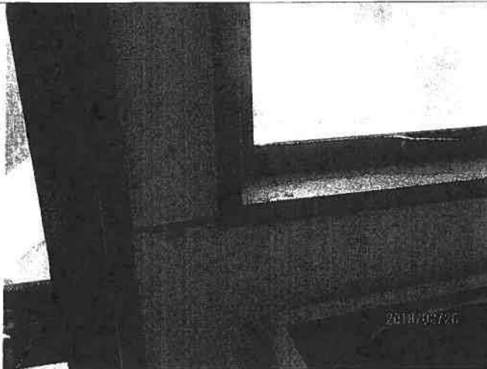
Gib wall lining separation in garage north wall
