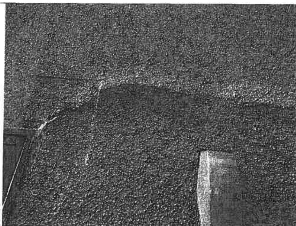
Localised bowing in plaster wall on north wall
