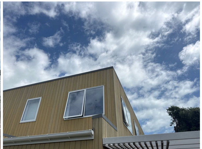
No soffits to most areas
