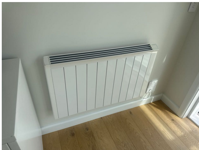
Electric heater installed
