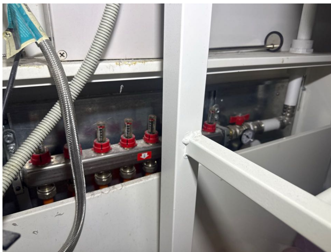
The manifold control for the in floor heating system is located by the hot water cylinder
