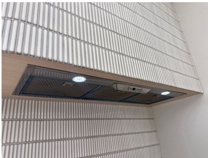
The range hood extraction unit is functioning
