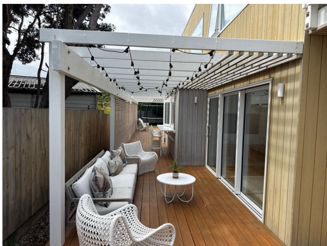
The timber pergola is structurally solid and secure. Rust affected fixings should be treated with rust converter.
