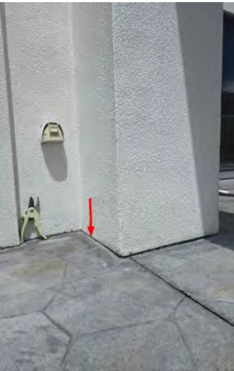
An example. Insufficient ground clearance.
