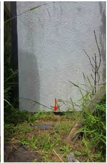
An example. Insufficient ground clearance.
