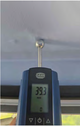
Under the west side flat roof where the paint has bubbled.
