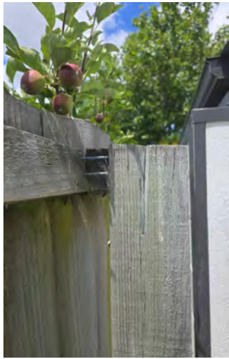
The north side fence railing is loose.
