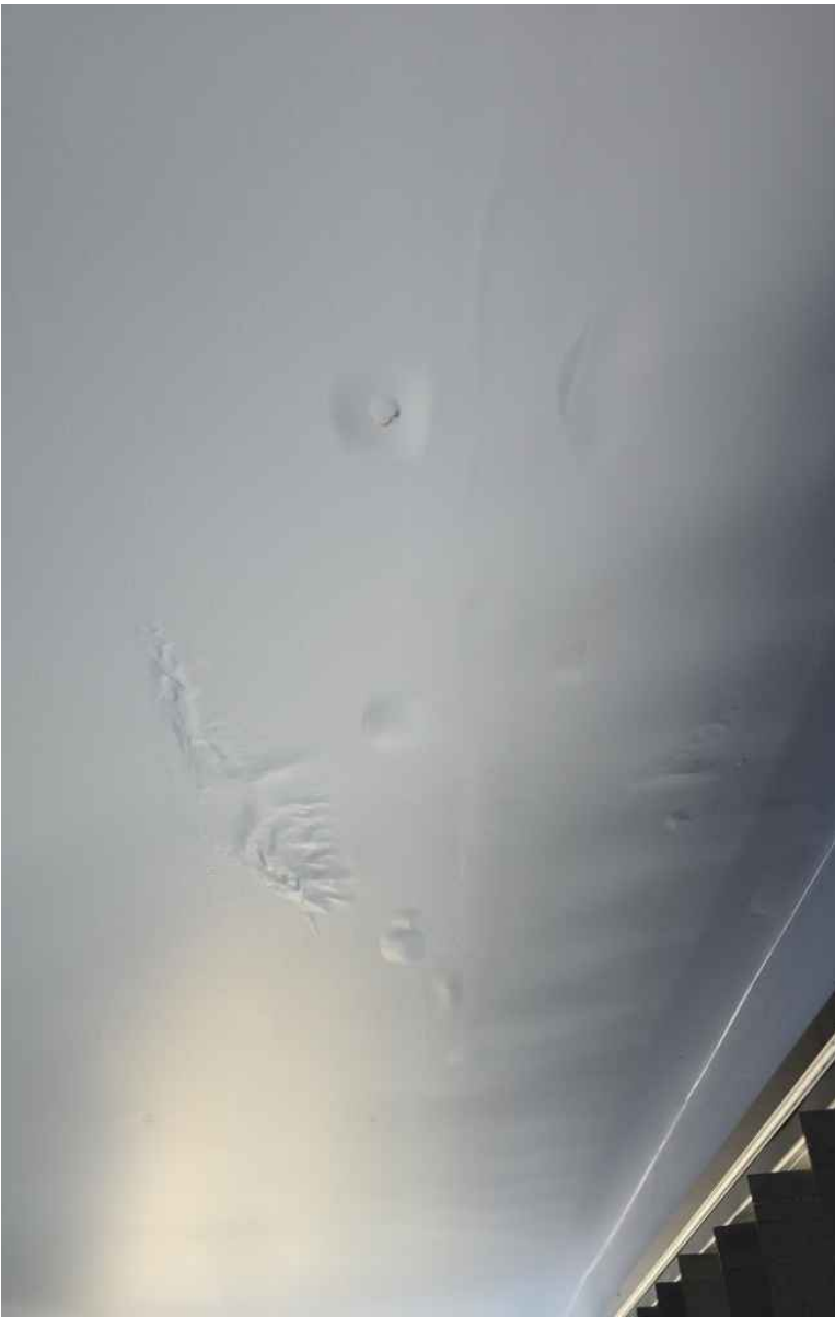
Bubbling of paint noted on the west bedroom ceiling under the flat roof.
