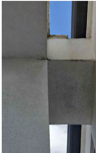
Minor cracking. This does not look to be of concerns as its outside the building envelope.
