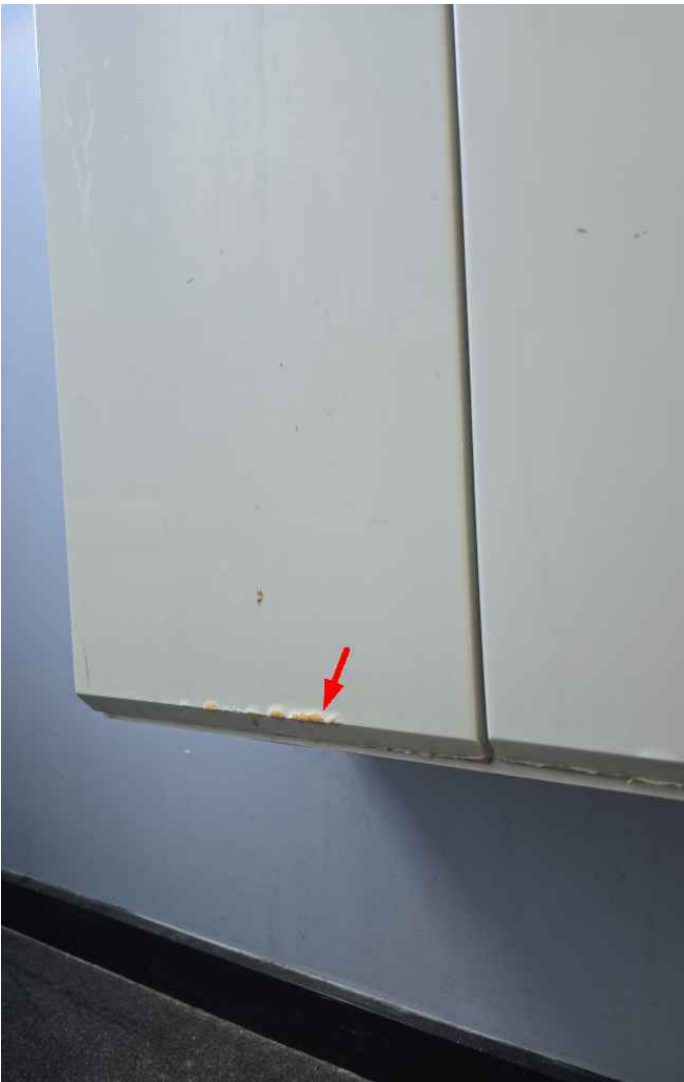
Water damaged cabinetry.
