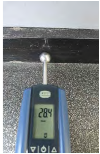
Under the upstairs toilet vanity.
