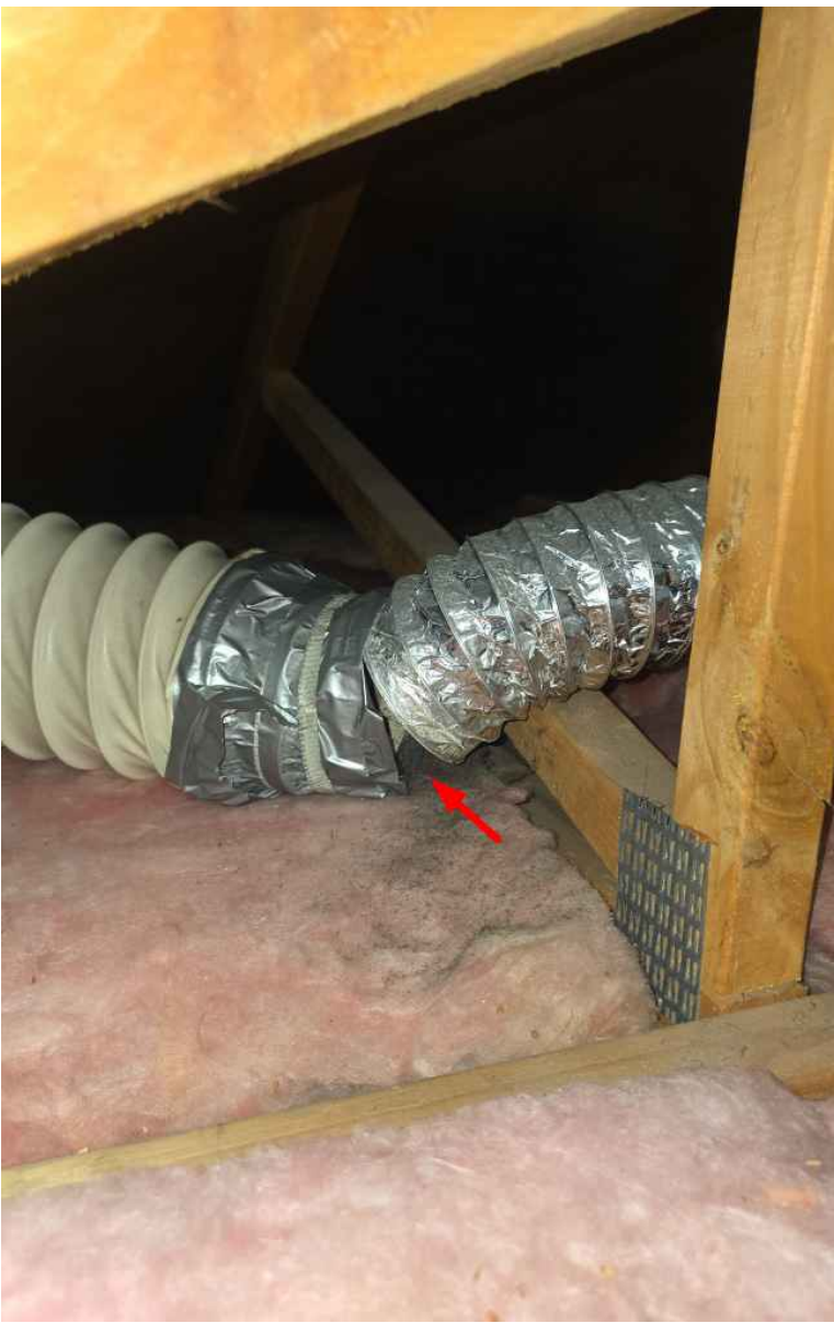
The bathroom ducting has come loose.
