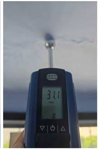
Under the west side flat roof where the paint has bubbled.
