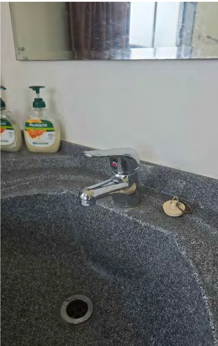
Loose bathroom tap.
