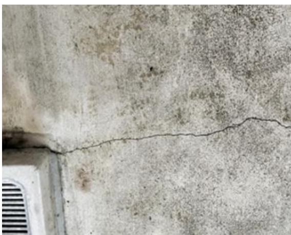
Crack in the garden path
