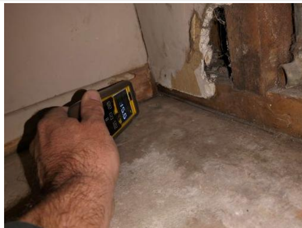
There's a hole in the wall inside the cupboard that houses the hot water cylinder. There is water staining on the skirting boards and plasterboard, this area tests in the dry moisture range
