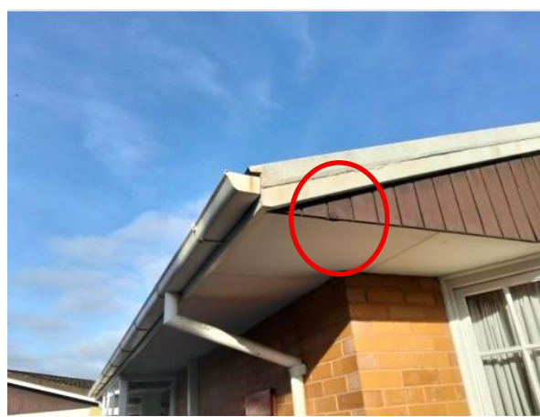
Damage to gable cladding adjacent to the driveway
