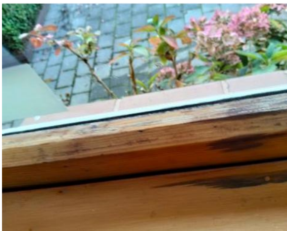
The timber windows are generally in good condition. There are some minor blemishes such as discoloration and fading of the coating
