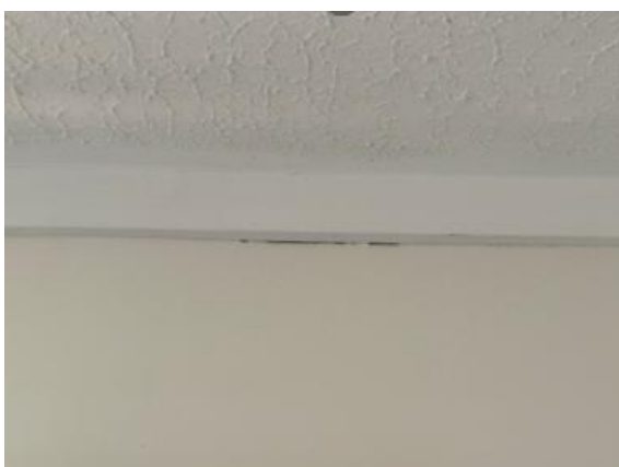
An example of a minor interior blemish, Paint cracking at the wall to ceiling junction in the living area
