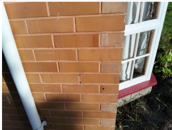
Brick cladding is generally in good condition; there are a few splashes of paint
