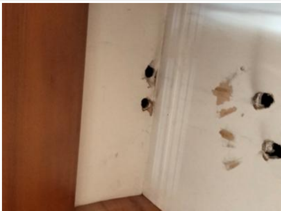
There are holes in the wall inside the entertainment cabinet in the living area
