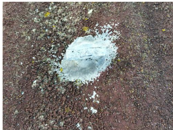
a redundant pipe penetration in the roof has been cut off and sealed
