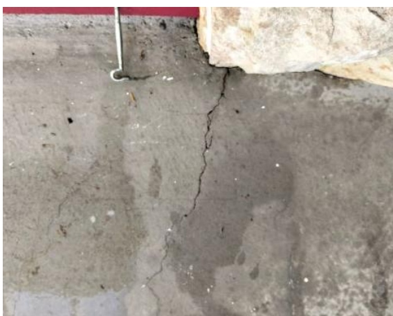
Crack on the concrete patio, there are a few minor insignificant cracks
