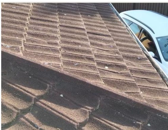
Denting on the roof tiles
