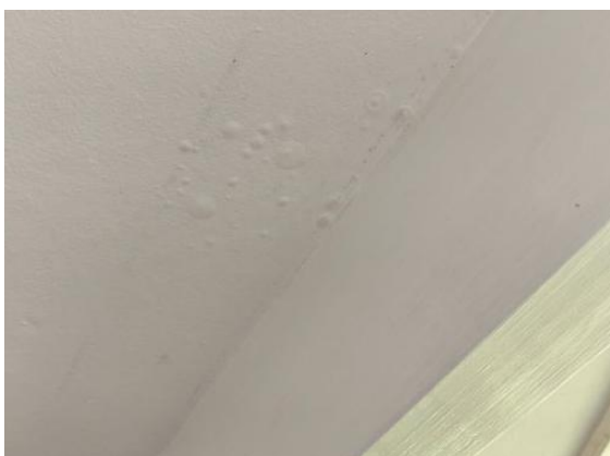
Paint bubbling on the soffit board near the main entrance
