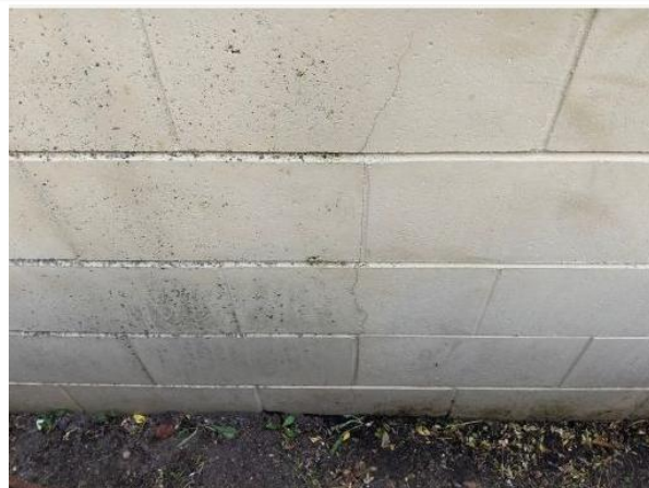
There are two vertical cracks in the blocks under the window at the back of the garage
