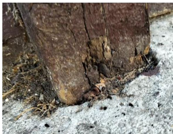
Deterioration at the base of a fence post adjacent to the driveway
