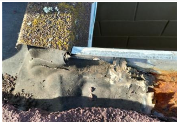
The transition from rubber membrane gutter to steel gutter is unconventional and does not appear well sealed,
