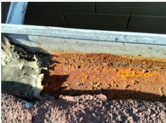
There is rust in the steel gutter just beyond the discharge point from the rubber membrane gutter
