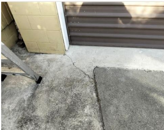
Crack and the concrete adjacent to the garage door
