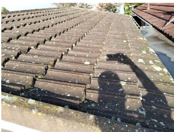
Lichen on the garage roof
