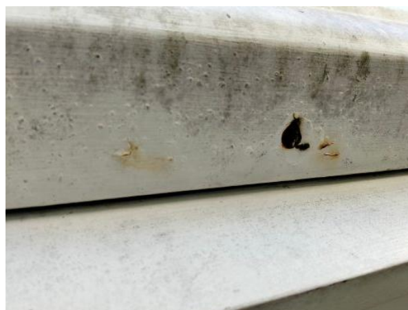
Rust on the underside of the gutter on the north side of the roof
