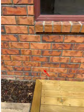
Minor crack to brick and mortar here.
