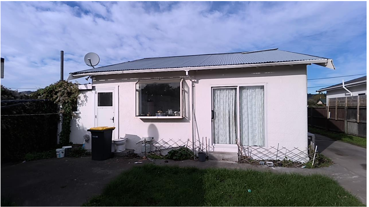
north existing vent Taken at 9:56 AM on Monday 28/04/2025
