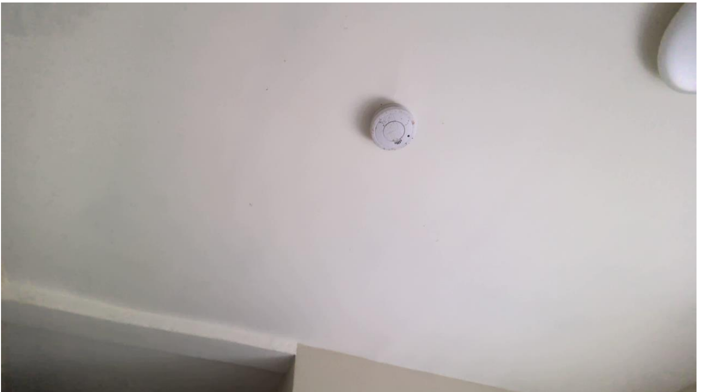
smoke alarms in place and tested Taken at 10:05 AM on Monday 28/04/2025
