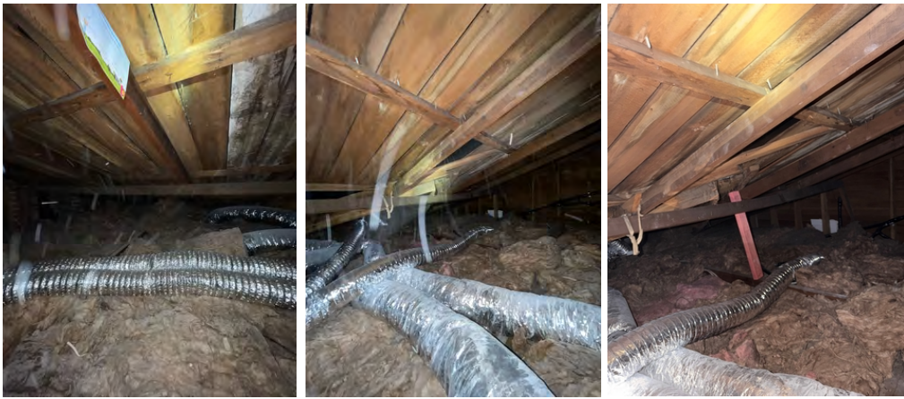
Extra vertical bracing has been added to help support the roof load.
