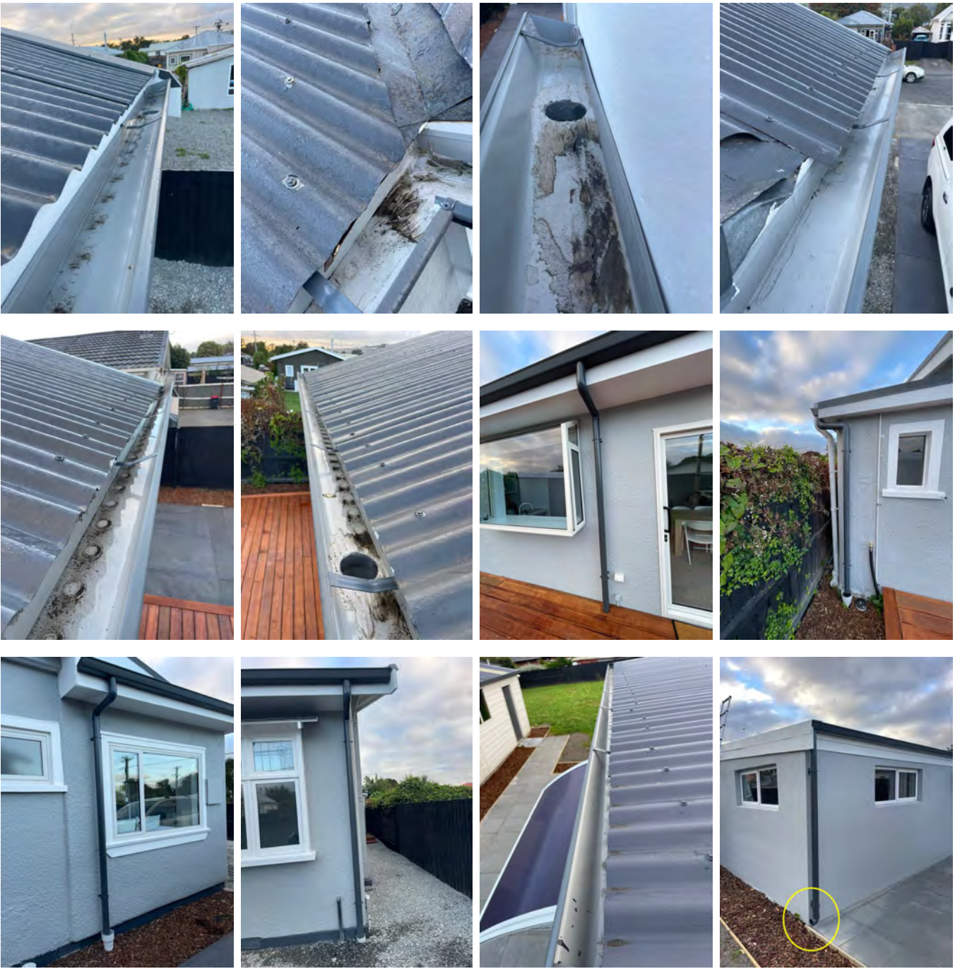
No stormwater riser noted for sleep out.
