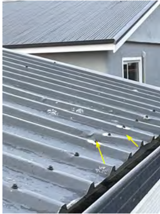
Some silicone repairs noted to some of the roofing fixings.
