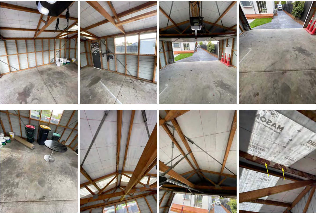
Example of moisture marks on the roof framing. Likely from previous popped roof fixings.
