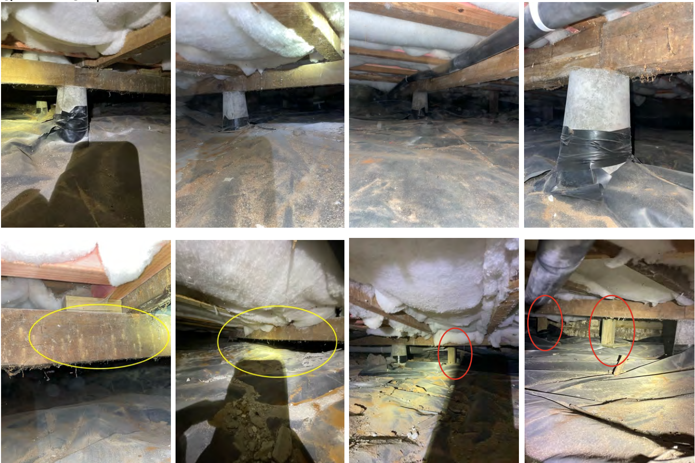
Example of borer noted on the subfloor framing. The client has provided evidence (photos and receipts) of recent borer bombs used in the subfloor area.
