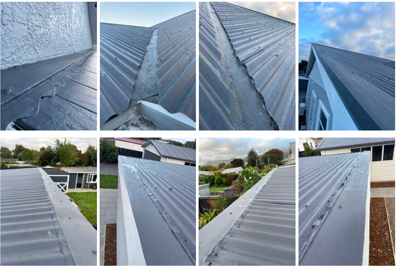
Flashings on the sleep out are aging but still look to be performing.
