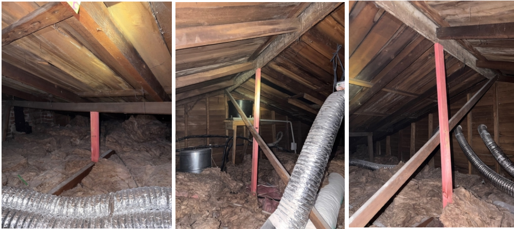
Extra vertical bracing has been added to help support the roof load.
