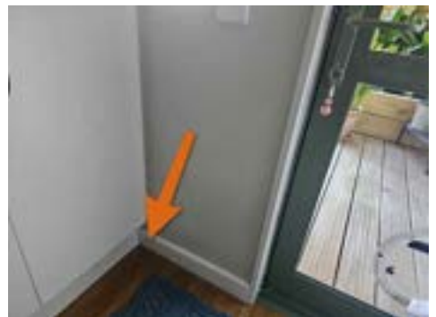
Laundry - 62.8% Elevated reading due to concrete nib wall
