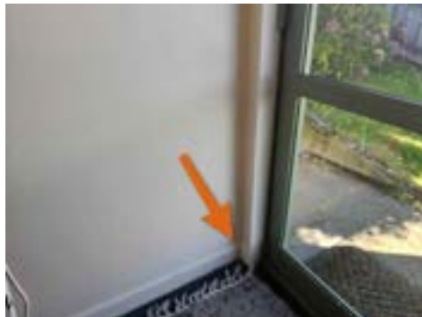
Garage - 23.6% Elevated reading due to concrete nib wall
