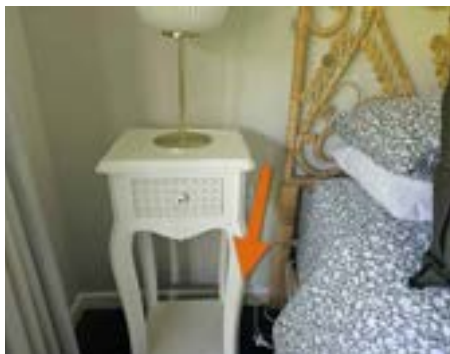
Corner Bedroom - 47.1% Elevated reading due to concrete nib wall
