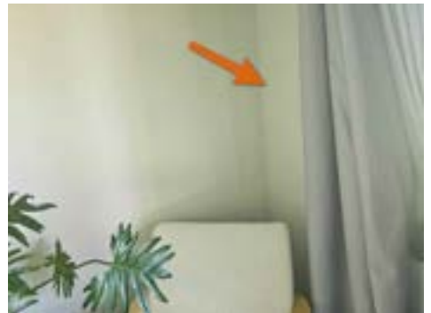
Corner Bedroom - 35.3% Elevated reading due to concrete nib wall or timber treatment
