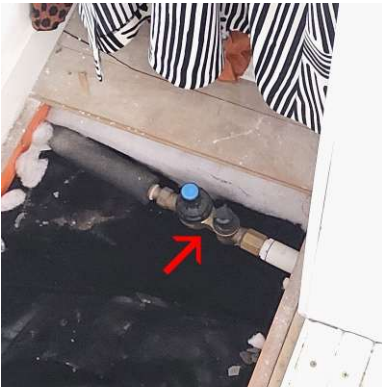
Shut off valve
