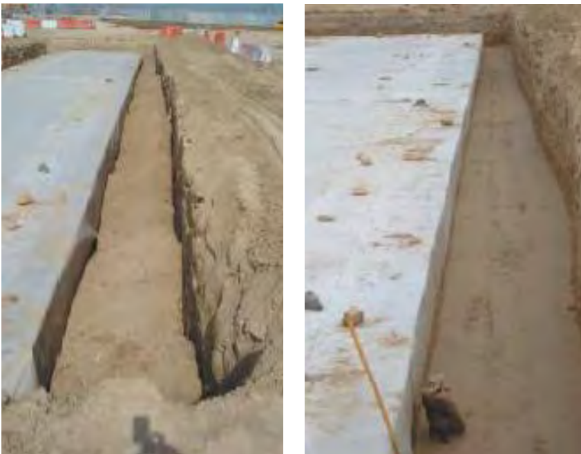
Fig. 22 Vibratory compaction of side backfill is always required, regardless of what backfill material is used.
