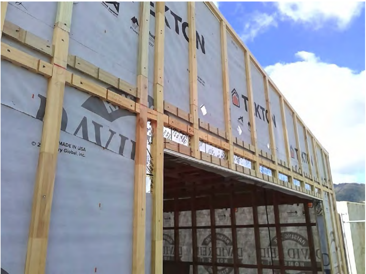
re battened gable wall. join fitted with fluted battens so cavity is maintained Taken at 11:42 AM on Wednesday 4/08/2021
