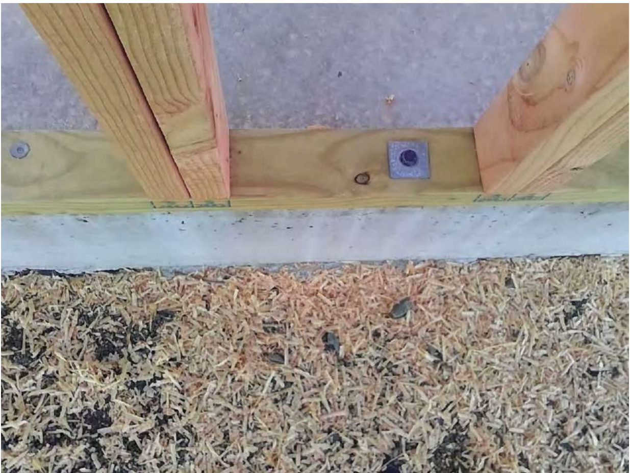
bluscrew bottom plate fixing to close to slab edge Taken at 8:36 AM on Wednesday 9/06/2021
