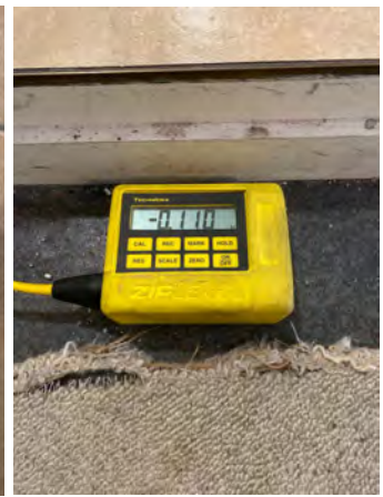
108mm step down into the garage.
