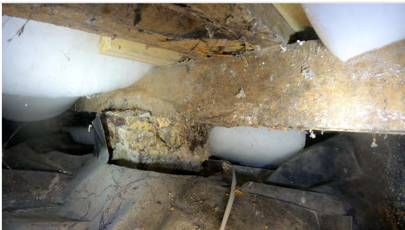
56: Jerry can pile with no connection.
