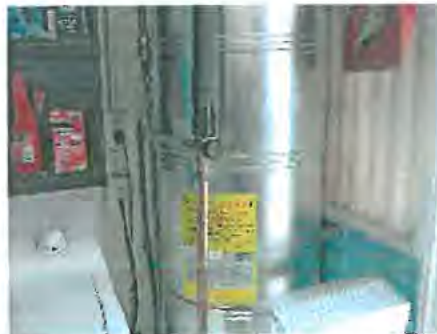
Water cylinder to laundry appears in good order.
