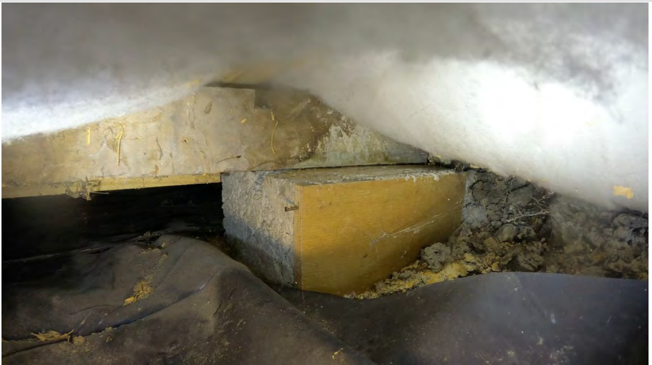
46: New concrete piles have been cast down this end of the home to support the bearers. No dampcourse has been used and no fixings are evident.
