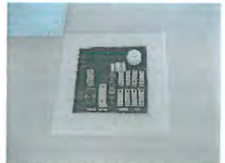
Fuse board to laundry appears in reasonable order.
