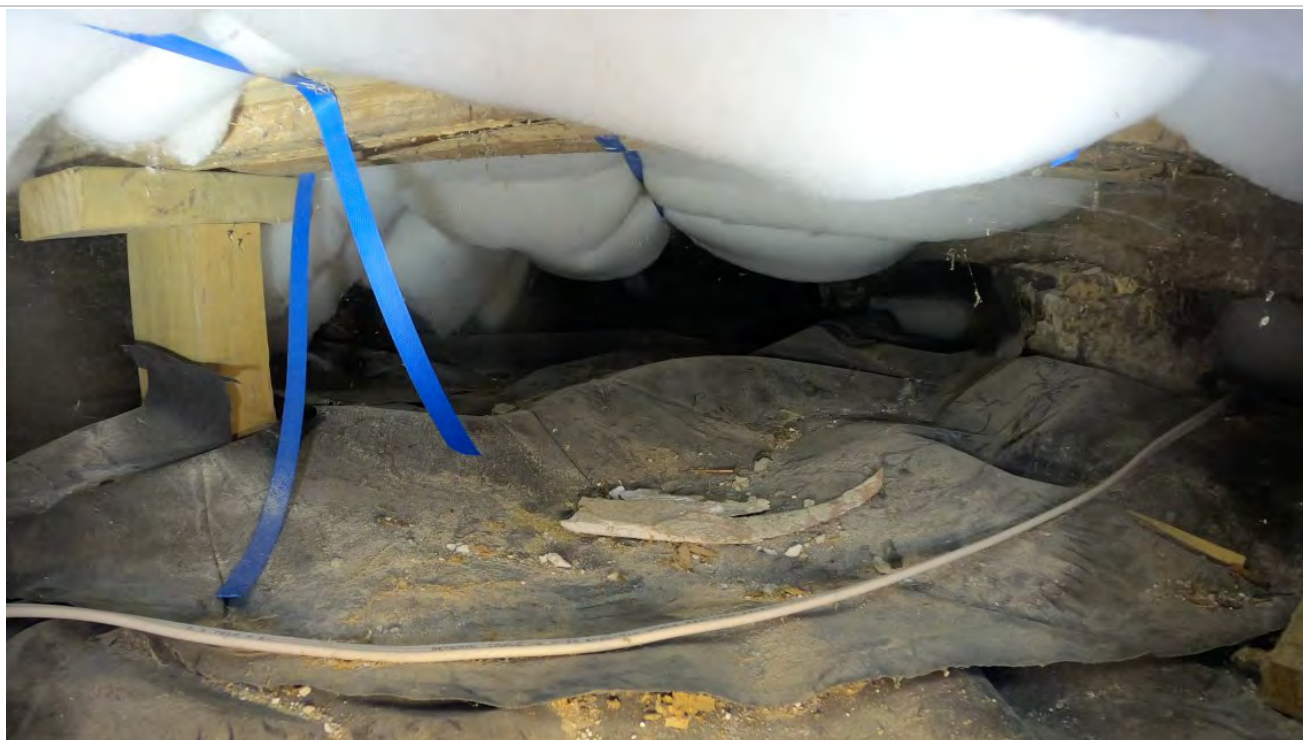
55: View of propping and the joist is cracked.
