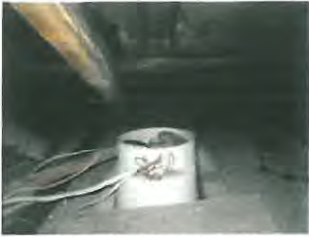
Bathroom extraction fan vents to the roof space.
