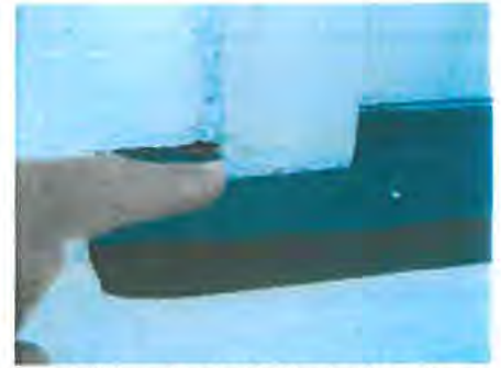
A little rot noted to the bottom of bedroom two window facing.
