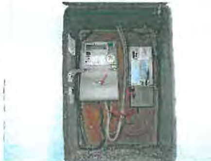
Meter box to outside wall.
