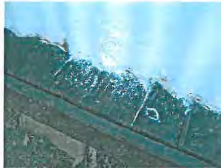
The conservatory deck is protruding outside the wall cladding.
