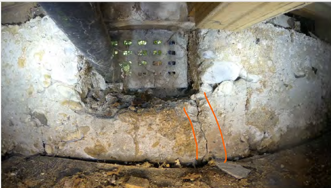
22: View of bearer meeting ring foundation with cracking. The foundations are average to poor quality type "B" rubble foundations. There has been extensive use of large stones in the aggregate. These can weaken the concrete and often create voids which affect epoxy repairs. It is not unusual to see fine cracking at the corner of vents and these existed pre-earthquakes however, the cracks we see are not just at the vents and are larger than would be expected. None show any sign of being repaired, so if the EQC scope of repairs says otherwise this would be important.
