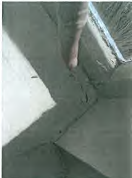
Rot noted to bedroom one window sill.
