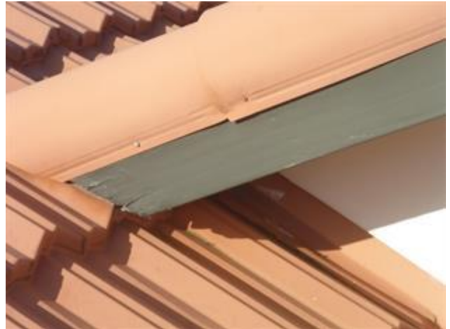
End grain deterioration
