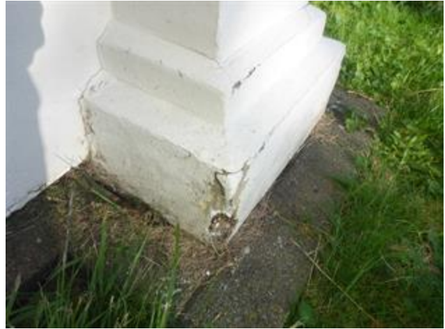
Impact damage front
