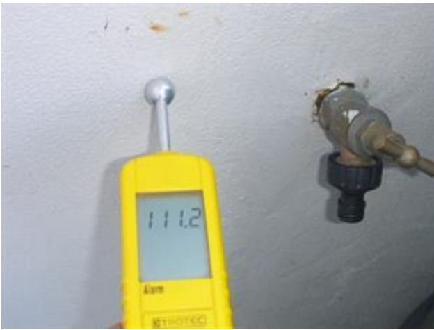
Rear tap high moisture levels
