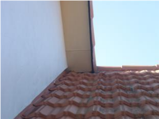
Fascia and soffit in contact
