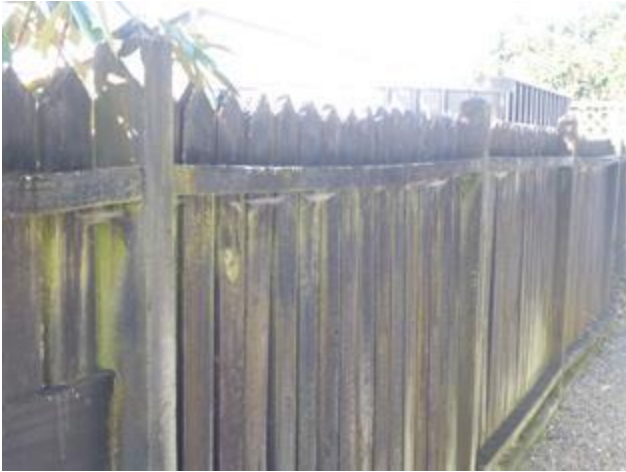
Post repair recommended
