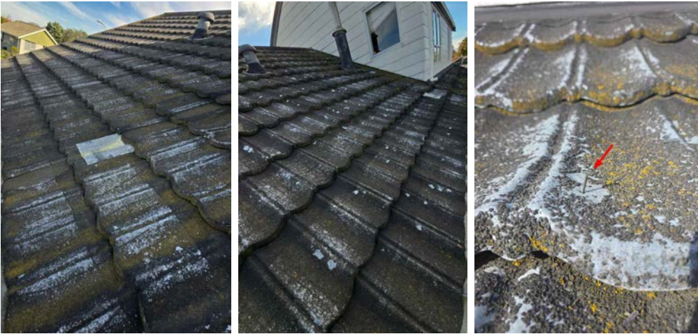
An example of a popped nail.
