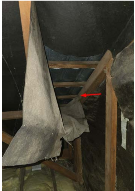
An area of roofing paper has ripped.
