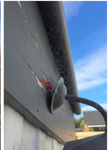
The external light fitting is loose.
