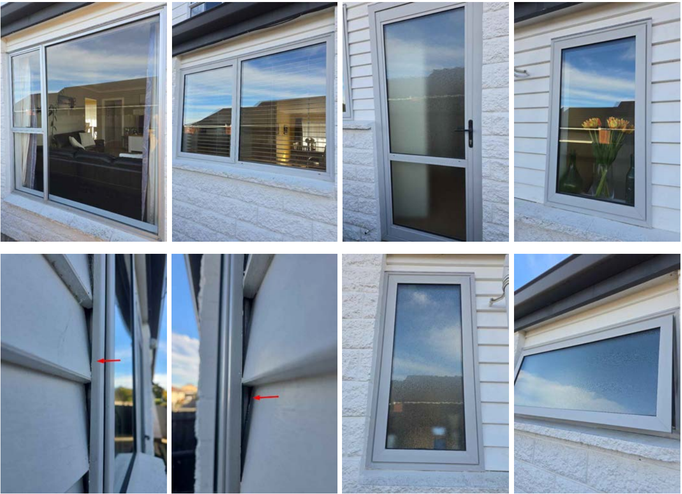
The laundry window is missing sealant against the cladding.
