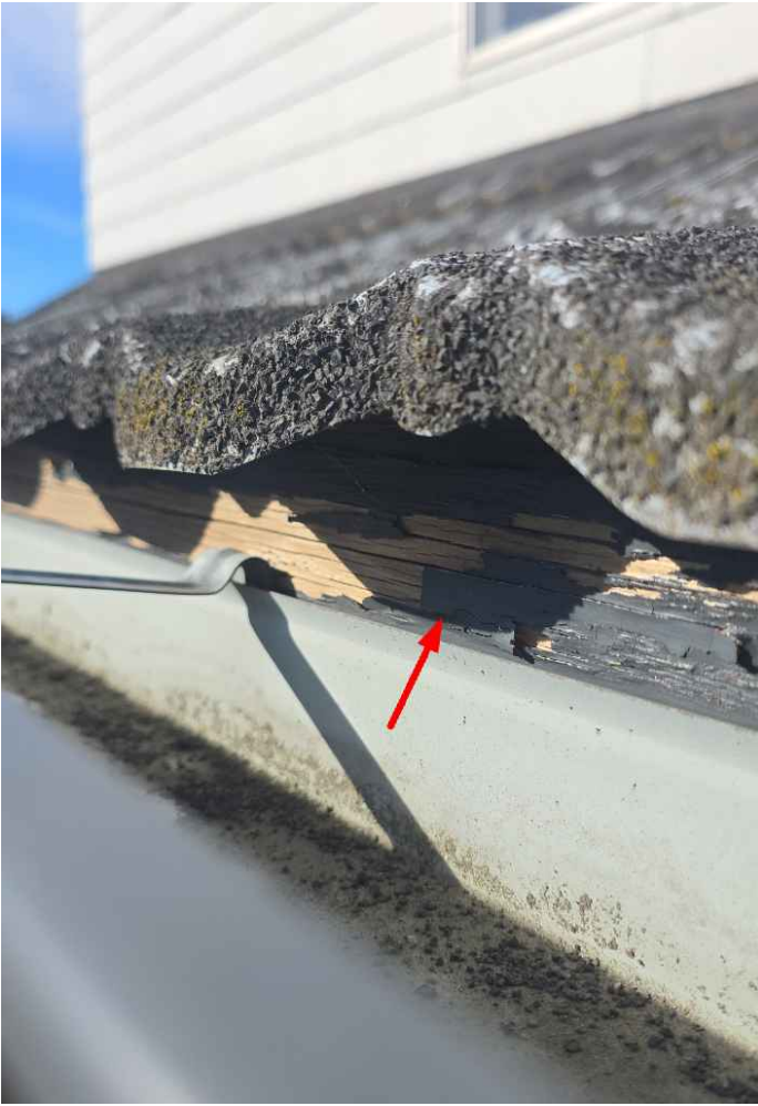
The paint is flaking along the fascia above the top level of the guttering.
