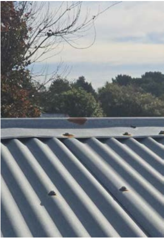
Isolated patch of surface corrosion noted.
