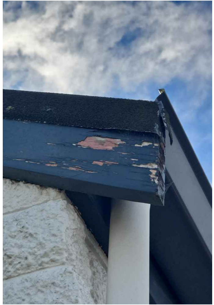
An example. Paint flaking noted throughout the fascia.
