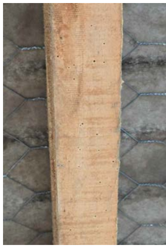
Borer holes noted within the roof structure.
