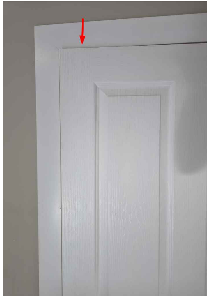
The downstairs northwestern bedroom door rubs along the framing.
