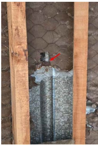
Rust noted to the ridge capping.
