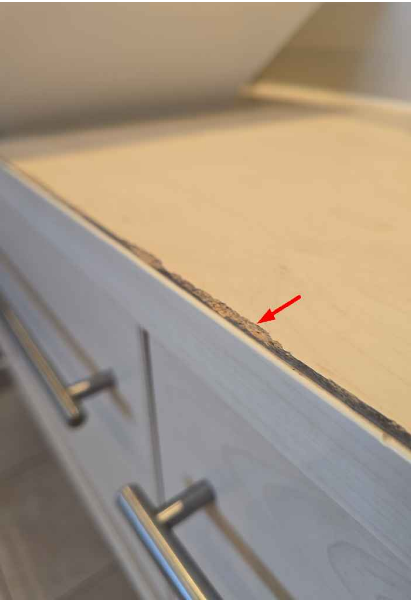
Water damage along the bathroom cabinetry.
