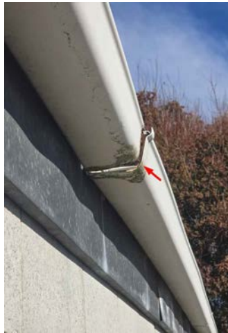
The west side guttering join has come loose.
