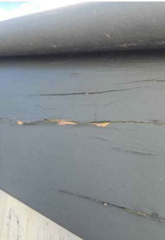
Minor paint flaking is visible throughout the fascia.
