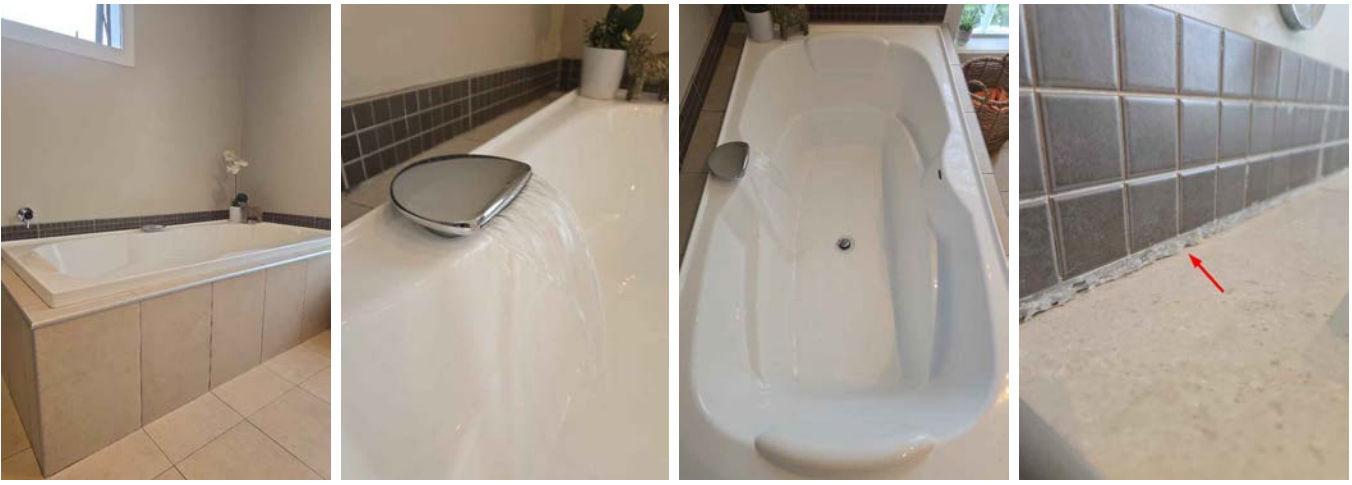
The sealant under the tiles could be tidied.
