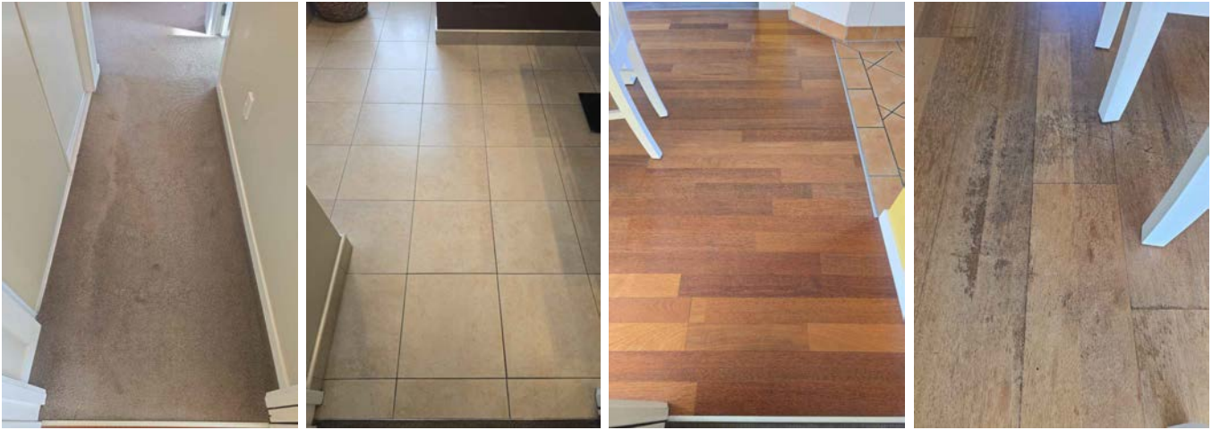
General wear and tear.
