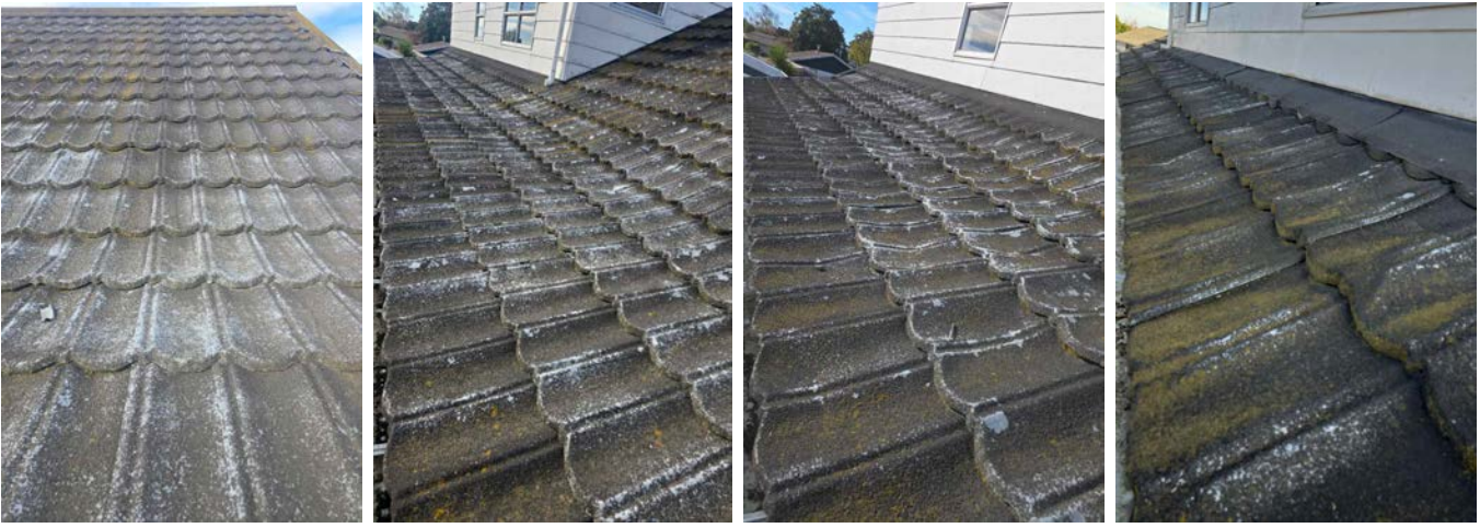
An example. Denting of the metal tiles is visible throughout the roof.
