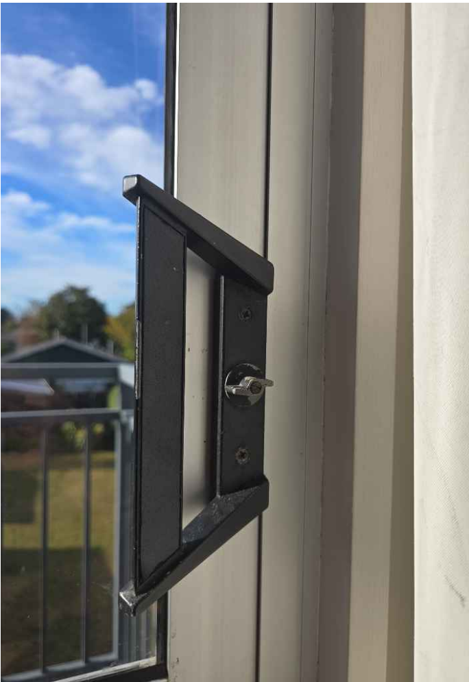
The upstairs balcony sliding door hardware is faulty.
