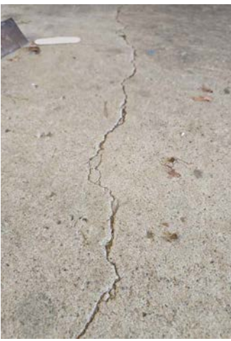
Cracking to the garage noted.
