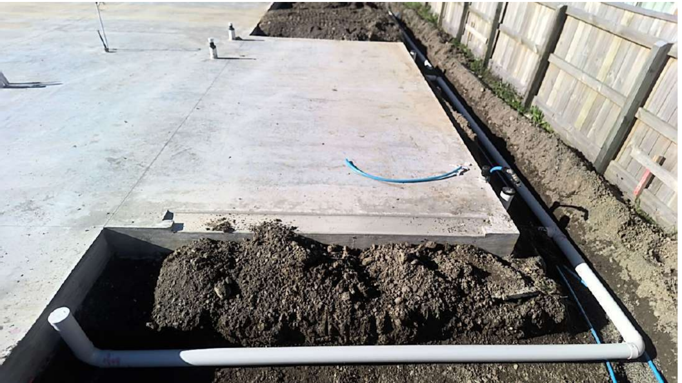
storm water Taken at 11:30 AM on Friday 23/05/2025
