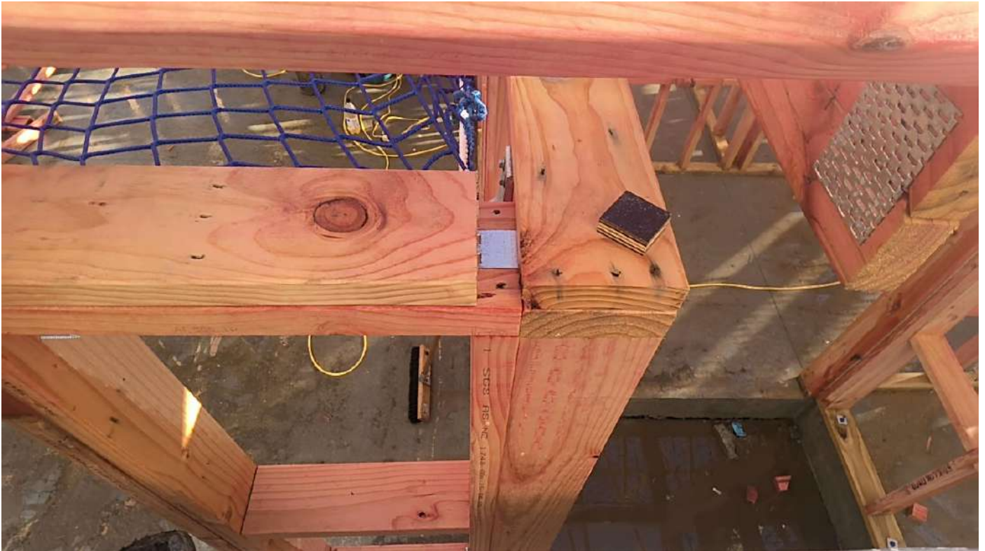
Adjacent to entry - indicative knuckle plate at intersecting frames Taken at 2:41 PM on Monday 14/07/2025
