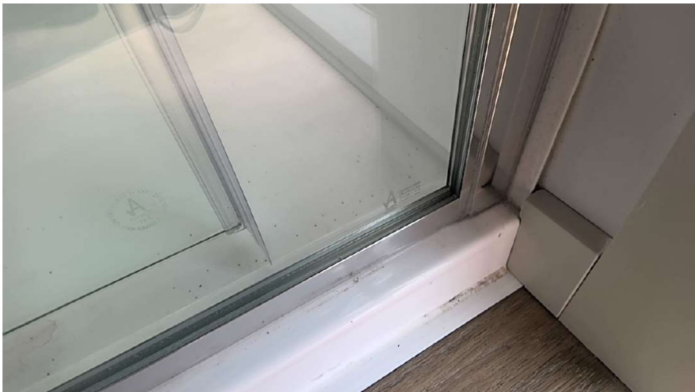
Safety glass to shower screens Taken at 10:46 AM on Wednesday 28/01/2026
