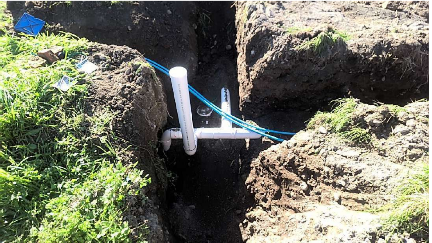
connection to lateral Taken at 11:29 AM on Friday 23/05/2025
