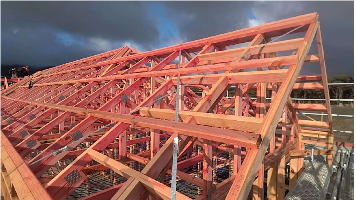
Bedroom wing West indicative roof straps and outriggers Taken at 2:39 PM on Monday 14/07/2025
