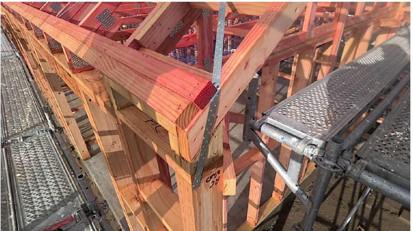
Bedroom wing West indicative roof strap end fixing Taken at 2:39 PM on Monday 14/07/2025
