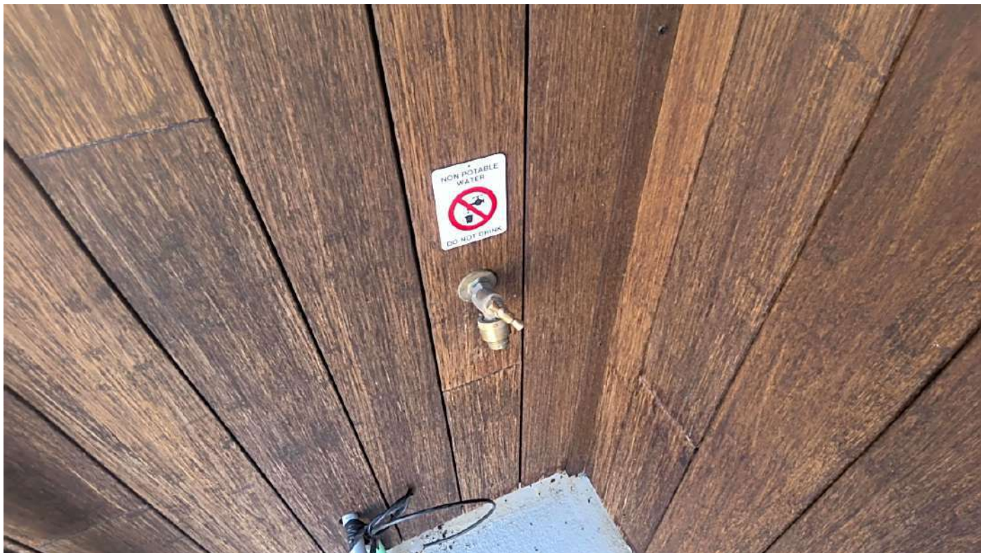
Non potable water signs
