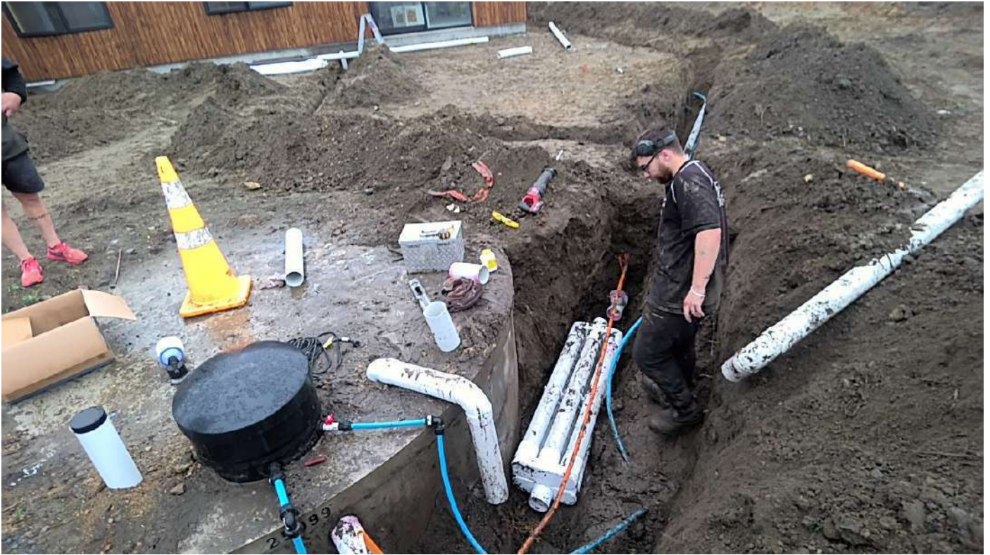
first flush bring installed Taken at 11:54 AM on Friday 10/10/2025
