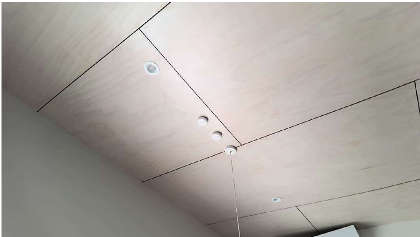
Smoke, and heat detectors in kitchen Taken at 10:38 AM on Wednesday 28/01/2026
