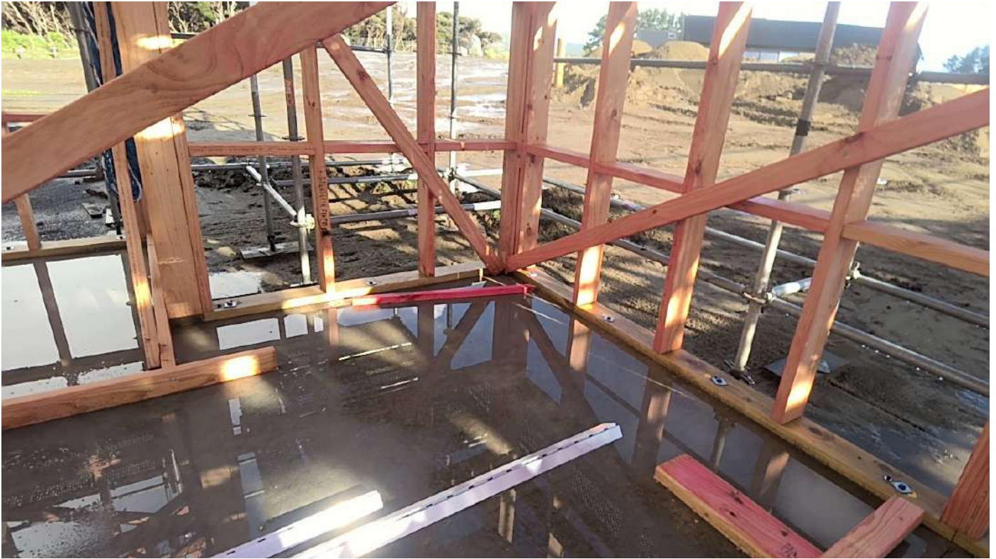
S/E corner - indicative BP hold downs - 140 framing Taken at 2:45 PM on Monday 14/07/2025
