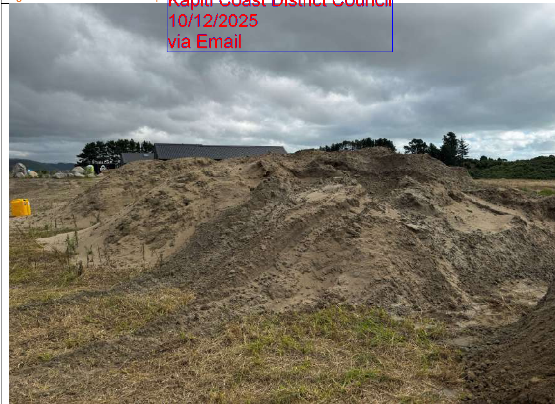
Figure 2: Stockpiled sands to be used as a FILL material are good quality and display minimal to no organics.
