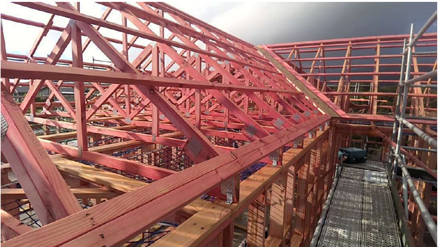
Bedroom wing East - indicative truss fixings CPC 40's Taken at 2:41 PM on Monday 14/07/2025
