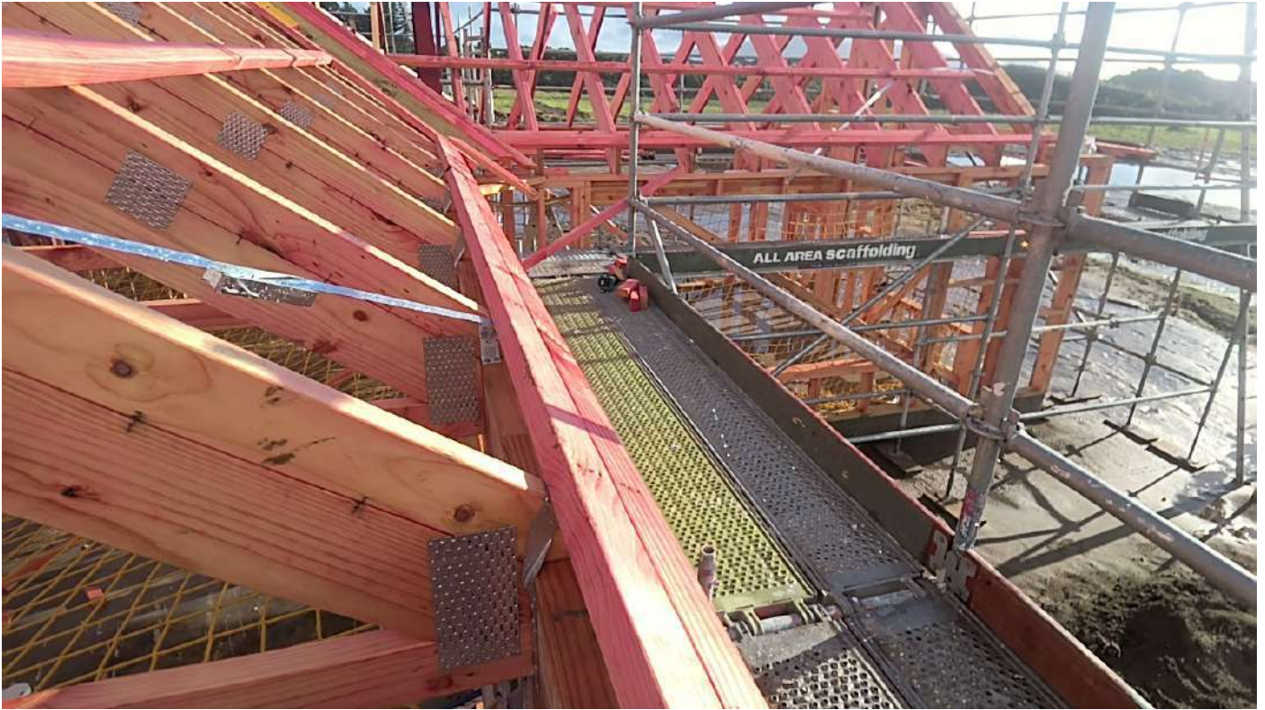
Garage N/W - indicative truss fixings CT's & CPC 40's Taken at 2:42 PM on Monday 14/07/2025
