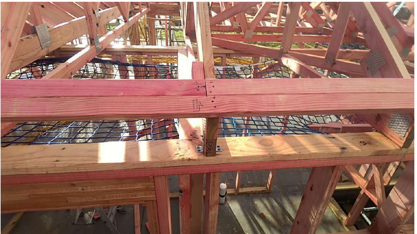
Over bathroom - indicative truss CPC 40's, purlin fixings and joint blocking Taken at 2:42 PM on Monday 14/07/2025
