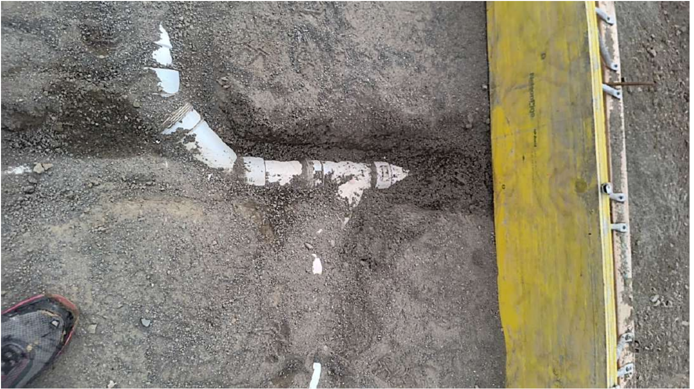
Typical junction Taken at 9:57 AM on Thursday 17/04/2025
