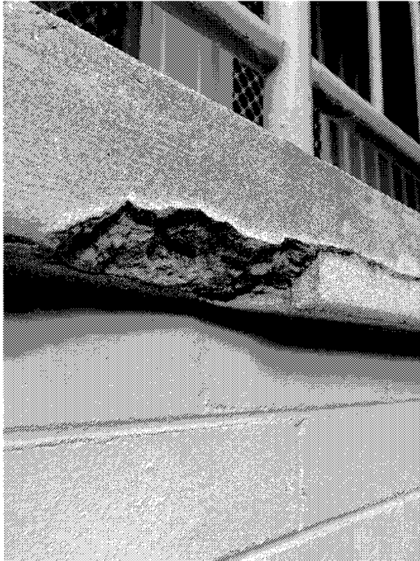
Figure 9 - Corrosion and spalling to lower walkway slab
