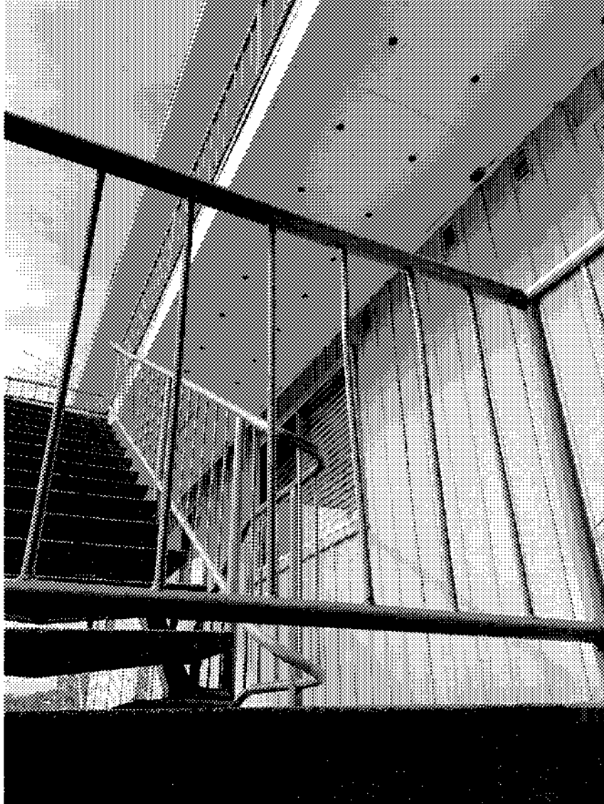
Figure 8 - View of underside of upper walkway from base of upper front stair
