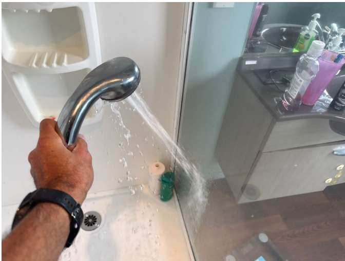
Good water pressure noted. No sign of current leaks from the shower frame during water testing.
