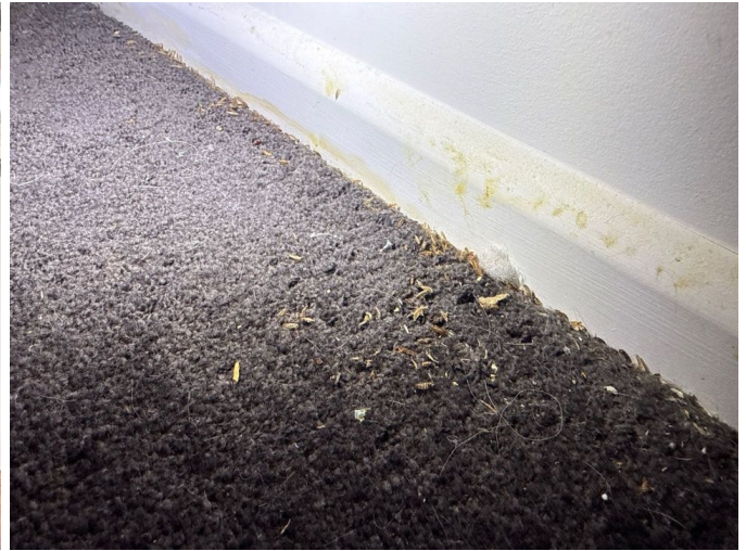
Carpet beetle activity by the hot water cylinder noted. A suitable chemical treatment should be applied to prevent further damage.
