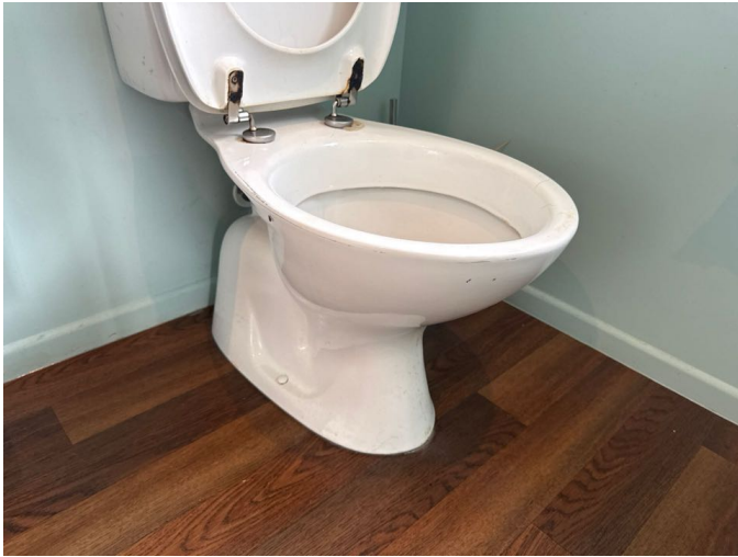
The base of the toilet is well sealed and secure. The toilet is in a functioning condition.
