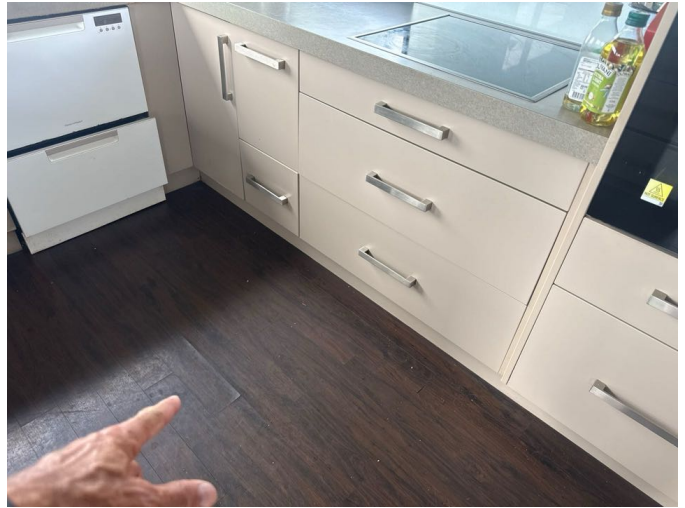
The vinyl plank flooring is starting to lift in areas and will need to be monitored.
