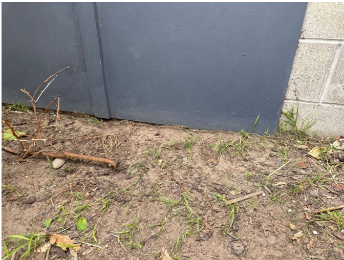
Ground levels should be lowered by the lemon tree The current building code requires a 150mm clearance between the internal floor height and the sealed ground and 225mm to unsealed ground. NOTE: The ground levels have been lowered since the original inspection.
