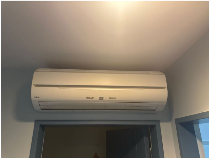
Heatpump/air conditioner to the ground floor hallway. Untested.
