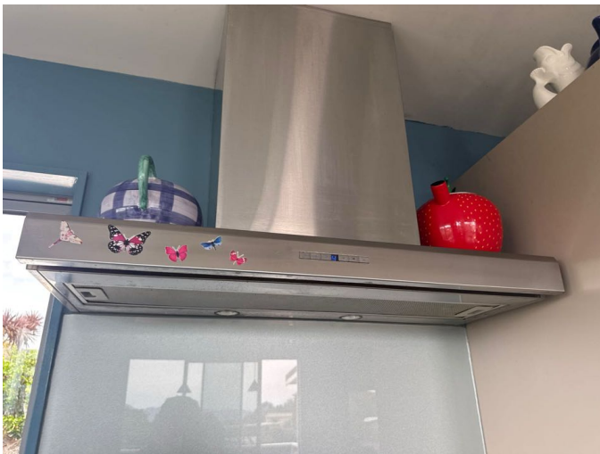
The range hood extraction unit is functioning
