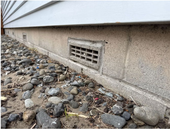
The concrete block ring foundation is in a typical condition for the age. No sign of cracking or significant stress.
