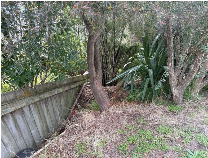
T.H.I.S is unable to comment on the condition of the fencing or retaining walls that are concealed by vegetation.
