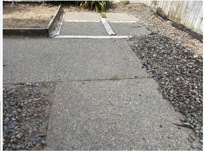
The paths are tidy and functional. Deterioration to the timber inserts at the southwest corner noted. Mainly cosmetic.
