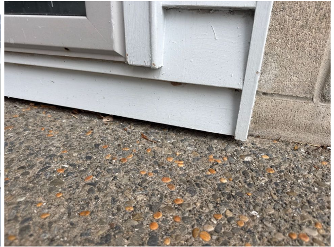
Example. Timber in close contact with the ground is at risk of premature deterioration and must be kept thoroughly sealed. Good current condition noted.
