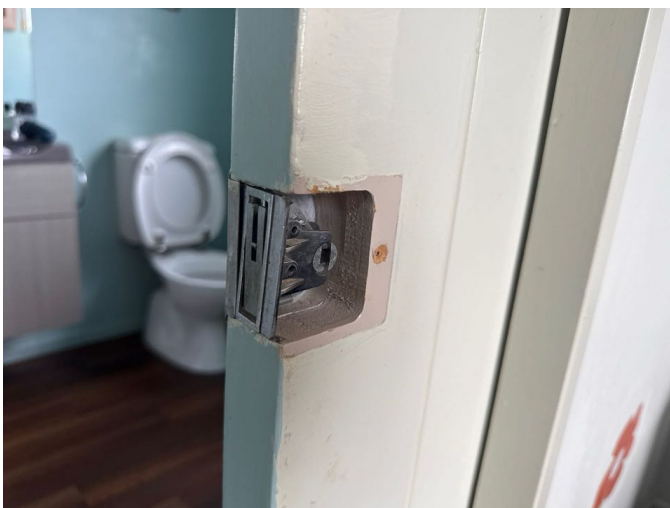
Part of the cavity sliding door handle is missing. The door is still functional as it is however it should ideally be replaced.
