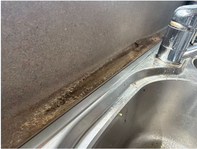
Wear to the bench at the back of the sink in particular. This is at risk of further damage. Thorough sealing improvements should be completed or the bench replaced in the near future.
