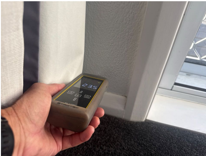
Moisture levels to the external walls were within the normal range at the time of inspection
