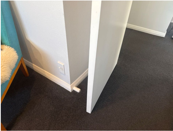
The internal doors are functioning well. Door stops installed behind the doors.
