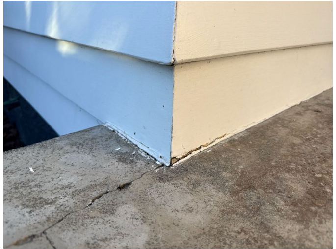
Timber in close contact with the ground is at risk of premature deterioration and must be kept thoroughly sealed. Paint improvements are recommended anywhere that surface wear is present.
