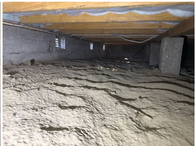
There was no evidence of significant water runoff to the sub floor
