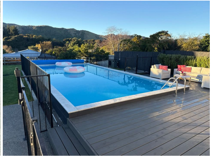
The condition of the pool and pumps etc were not checked as part of this inspection process. The fence is secure and the security gate is functioning. The timber deck is in good condition.
