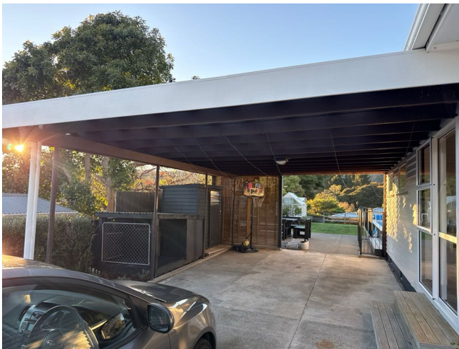
The steel and timber carport structure is showing no evidence of imminent structural issues
