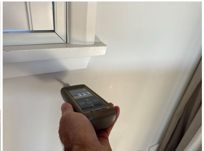
Moisture levels to the external walls were within the normal range at the time of inspection
