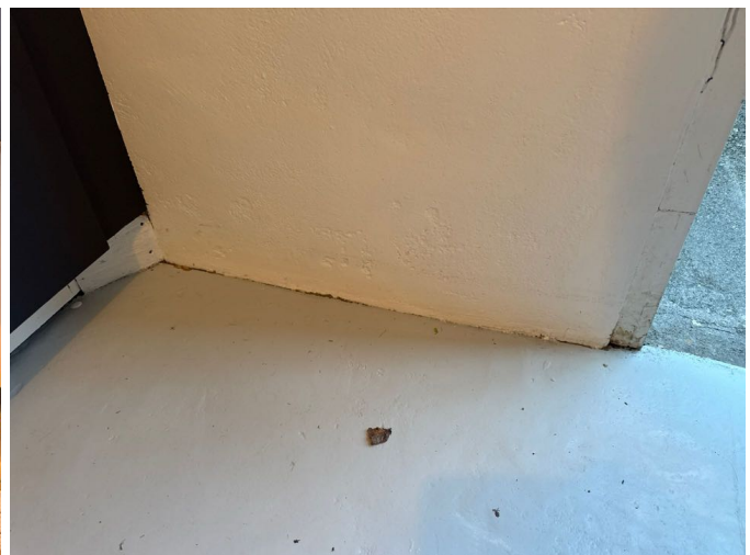
Concrete walls and floor noted. These areas could not be moisture scanned. The painted interior is tidy.
