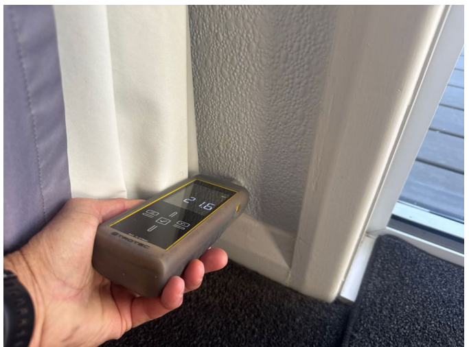
Moisture levels to the external walls were within the normal range at the time of inspection
