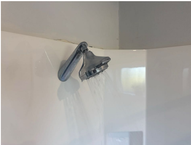
Good water pressure noted. There is some early stage paint deterioration around the top of the wall above the shower frame which will require attention in the near future.
