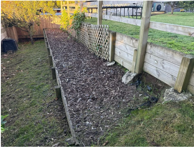
Solid timber retaining walls to the east side. No sign of significant movement or damage.
