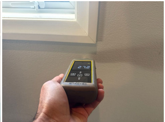
Moisture levels to the external walls were within the normal range at the time of inspection
