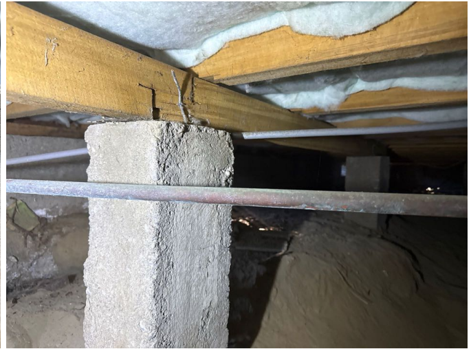
The concrete piles are solid at the time of inspection. Galvanised wire connects the bearers to the piles and anchors the structure to the ground.
