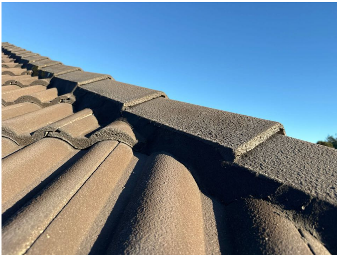
The ridge caps tiles are sealed with mortar which is prone to cracking. Well maintained current condition noted. Periodic monitoring is required. When cracking becomes evident, engage a roof rejuvenation professional to re-point any areas of concern.
