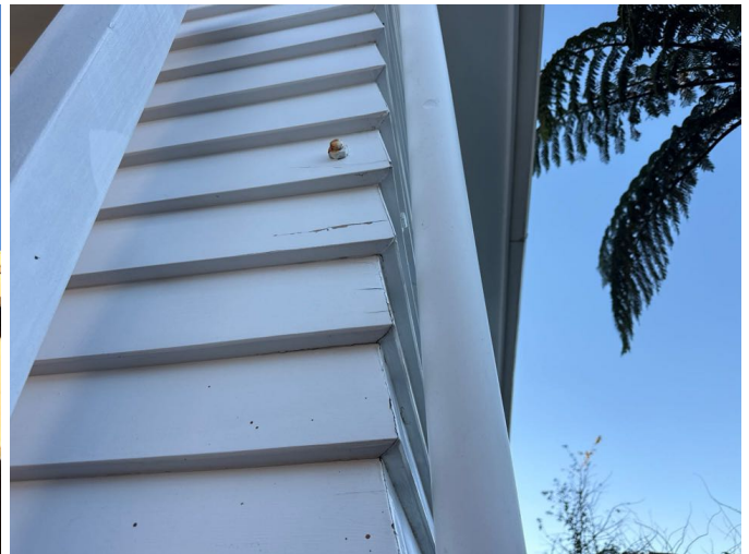
Example. Early stage surface deterioration to the paint in some areas.
