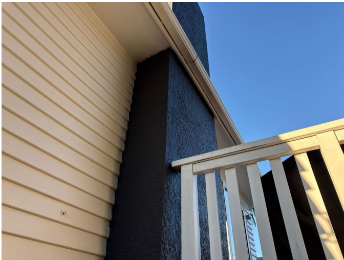
There was no evidence of damage or movement to the concrete chimney
