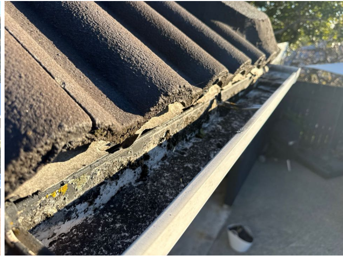
The spouting is in an average condition and was clear. The effectiveness of the spouting will need to be checked during rainy periods. Due to the dry conditions that were evident on the day of our inspection we cannot comment on any leaks that maybe evident to the spouting or down pipes.
