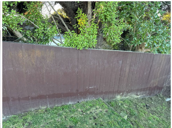
North side. Due to the age of the home some of the materials used in the fences construction may contain Asbestos. Safe in an inert state (well encapsulated and not disturbed) but if any repairs are needed to areas that may contain Asbestos then there are certain health and safety precautions that must be followed.
