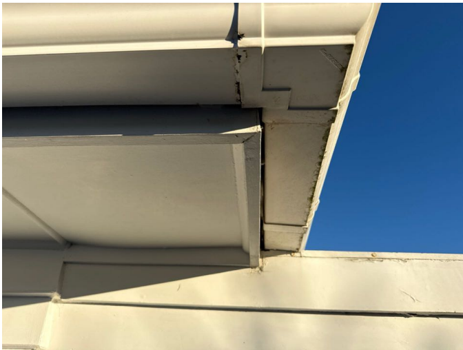
Good paint quality to the timber fascia and fibre cement soffit linings
