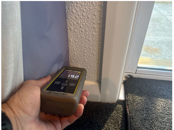
Moisture levels to the external walls were within the normal range at the time of inspection
