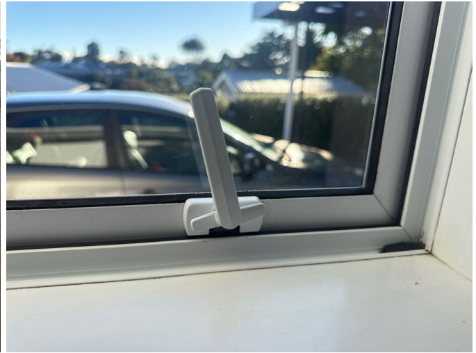
Part of the window hardware is missing from the framing which prevents the window from sealing effectively. These can be retro fitted which will help improve the seal. Maintenance recommended.
