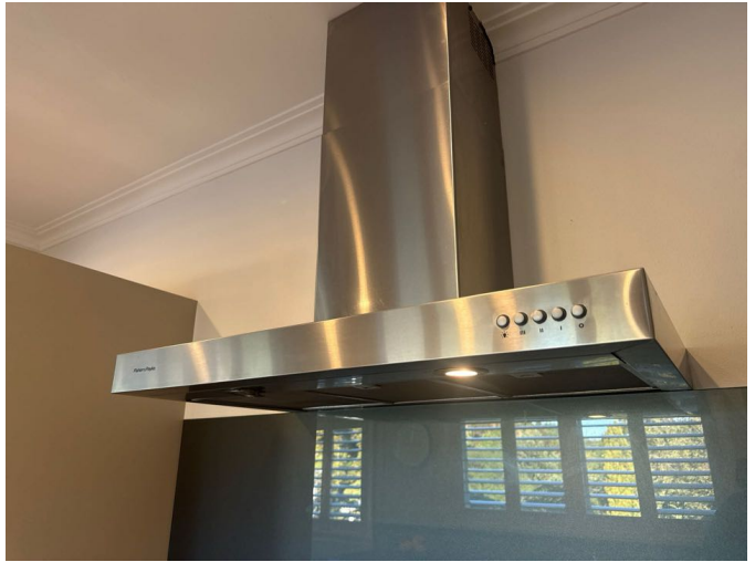
The range hood extraction unit is functioning
