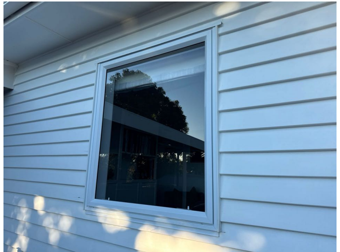
The typical single glazed aluminium window detail consists of head and sill flashings and timber scribes.
