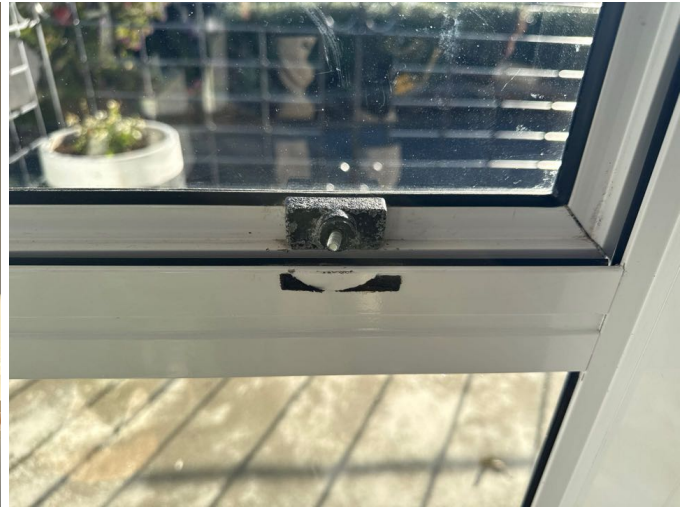
The broken window handle should be replaced
