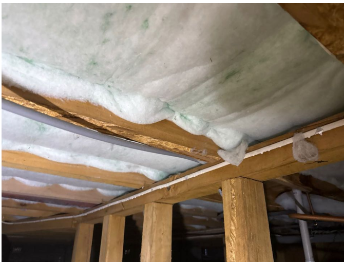
Polyester insulation is installed in the sub floor. There is no labelling present to indicate the R-Value of the material.
