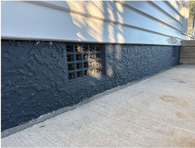
The concrete ring foundation is in a typical condition for the age. No sign of cracking or significant stress.
