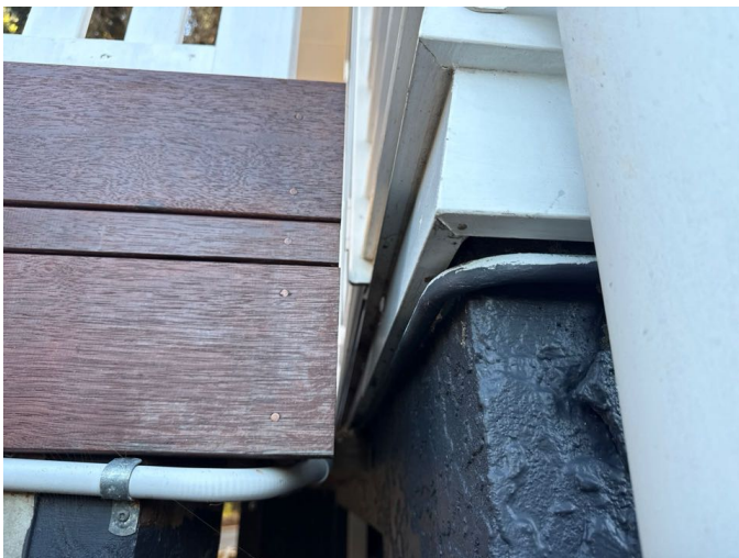
Good clearance between the deck and the cladding which will allow water to drain away.
