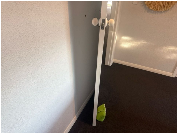
The internal doors are functioning well. Door stops should be installed where missing to prevent the risk of damage to the wall linings (some damage present).
