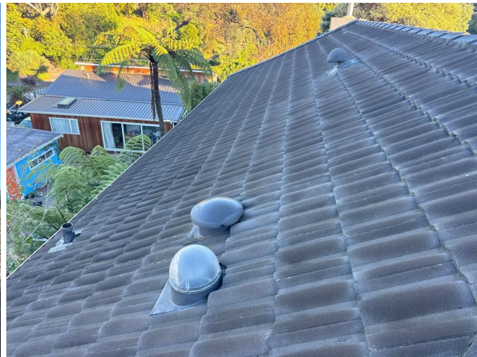
The roof penetrations were effectively sealed at the time of the inspection
