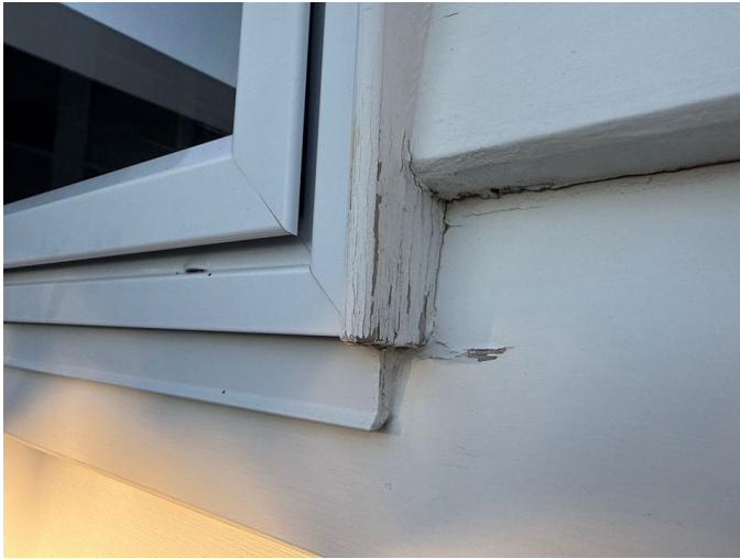
Paint deterioration to the timber scribes
