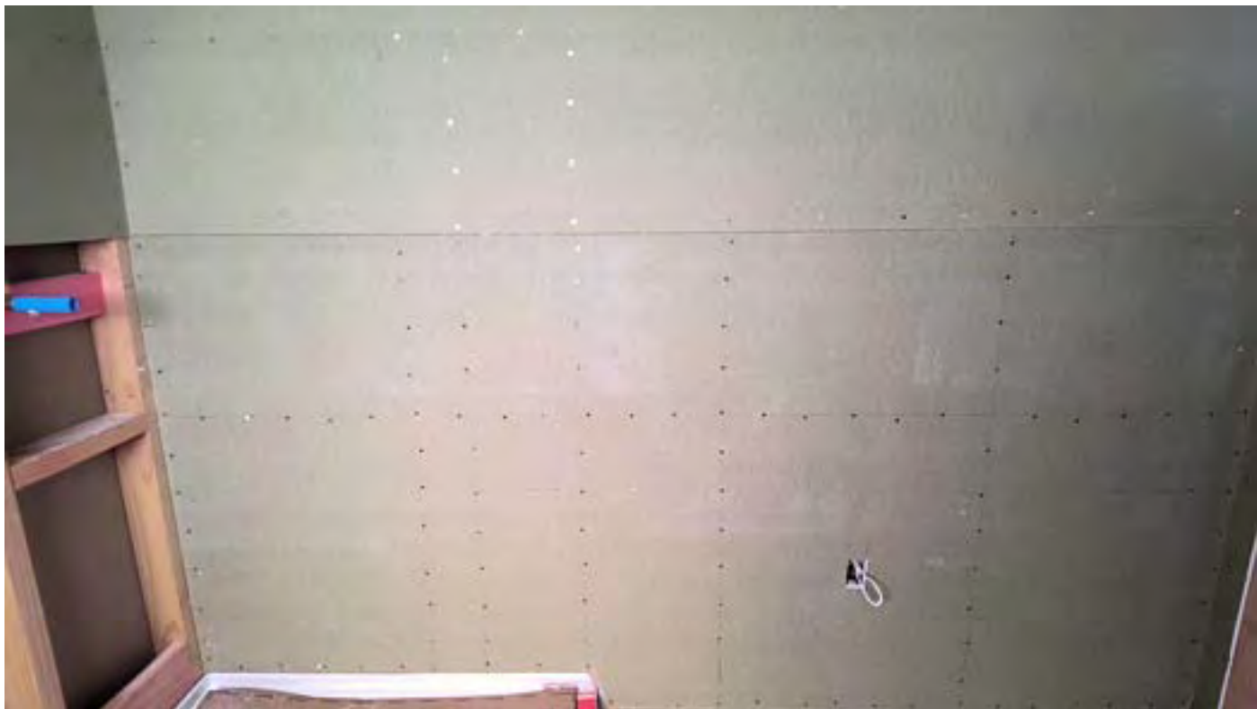
main bathroom - Note: acrylic shower units - Aqualine fixed off for tiled half height wall beyond shower Taken at 10:45 AM on Friday 8/09/2023
