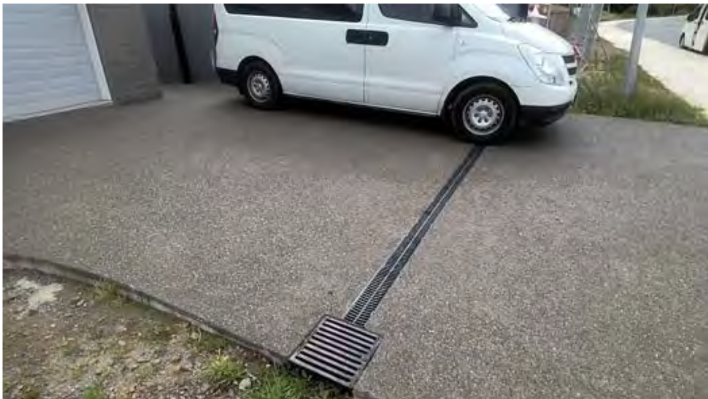
Dtrip drain in driveway Taken at 9:54 AM on Friday 20/12/2024
