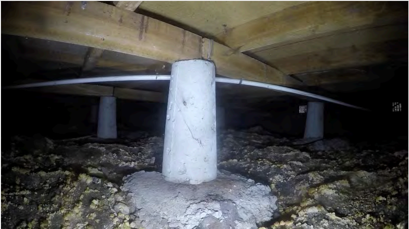
28: Pile with bearer join. There is significant yellow mold growing beneath this home.
