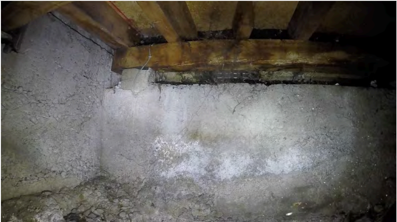
6: The home has outside bearers supported on concrete blocks embedded into the foundation and connected with stapled off wire. The outside bearers show signs of water damage in several areas along the foundations.
