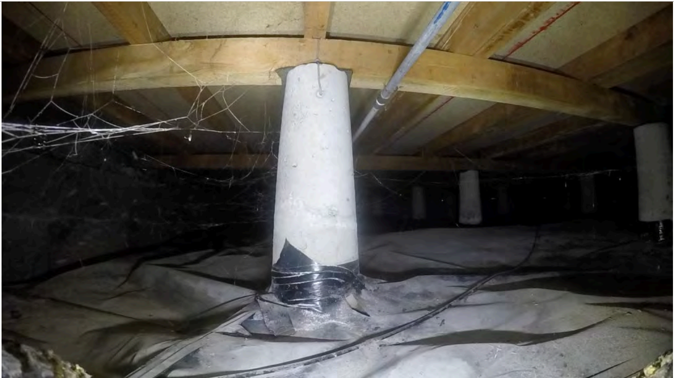
8: All piles appear to have their original connections, however there are several piles that the stapling has not been carried out correctly.
