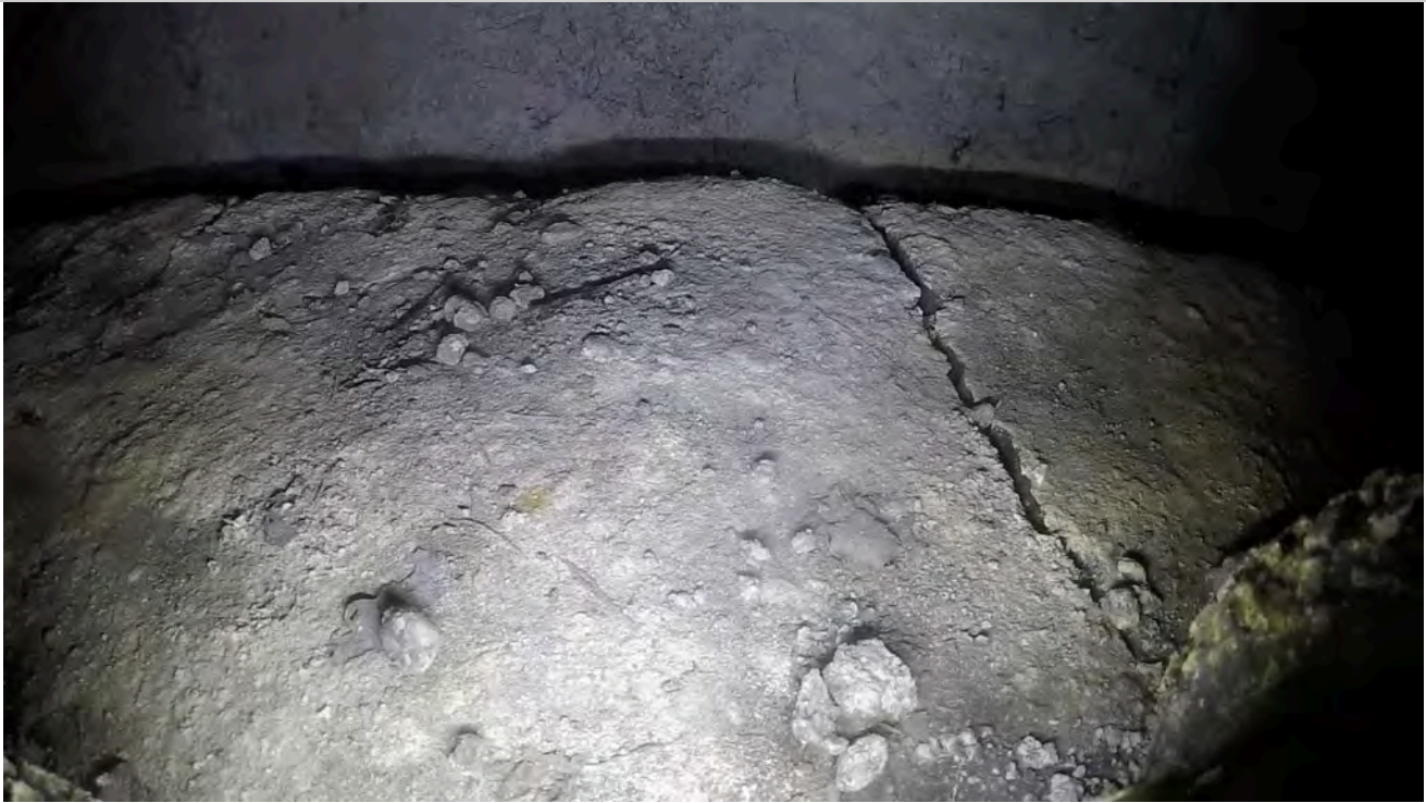
9: Large ground crack heading towards the foundation.
