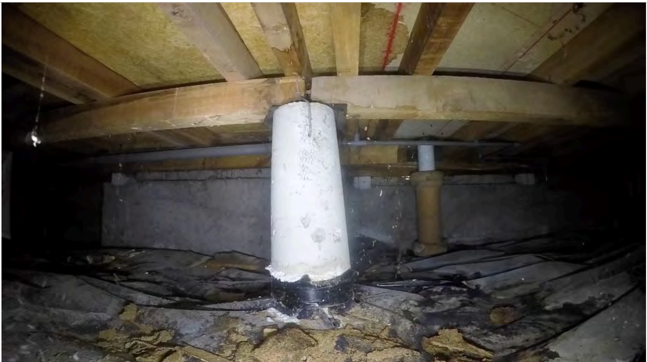
38: There are indications of an above floor water leak here and the timber is showing signs of water damage.
