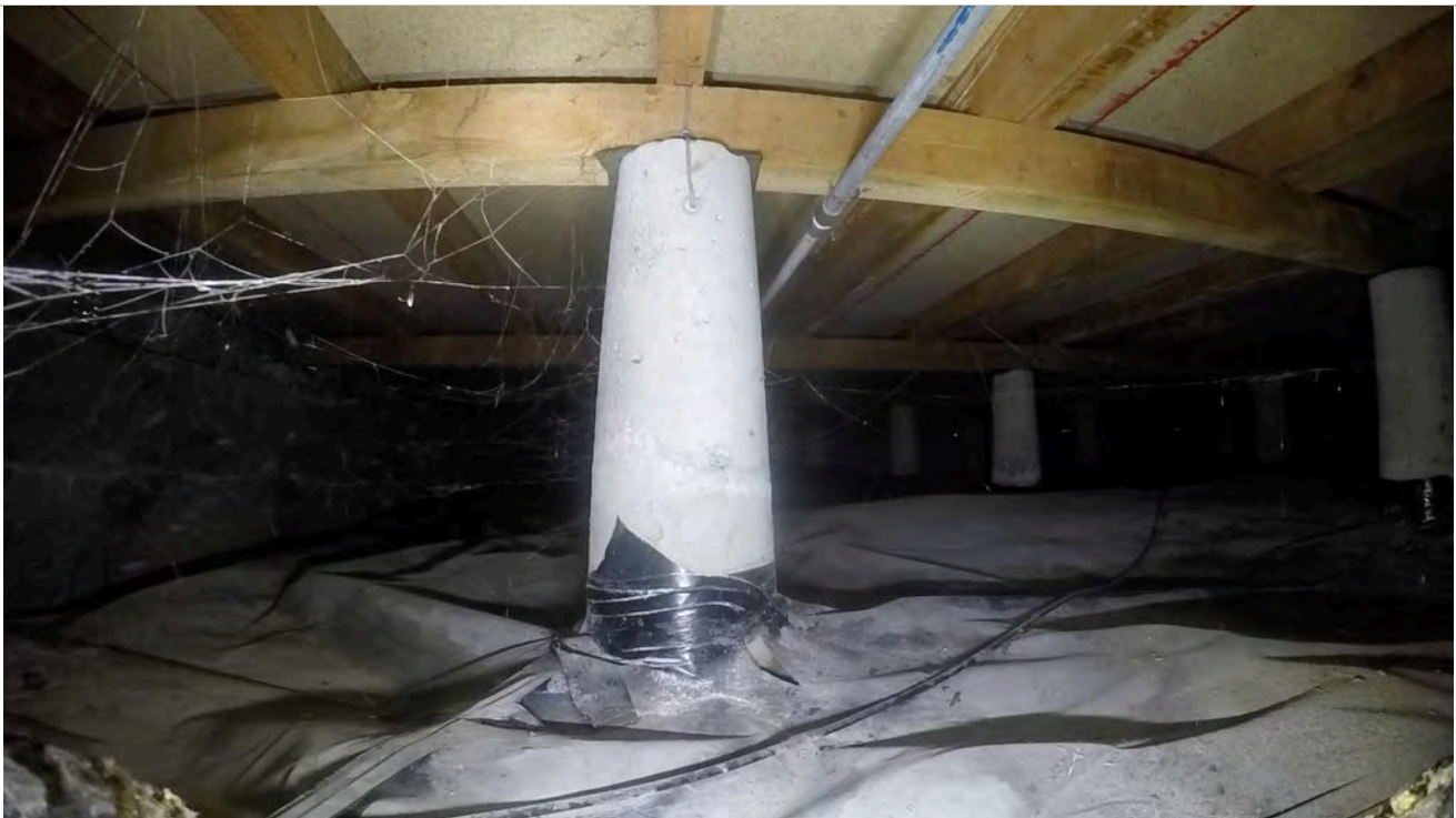
8: All piles appear to have their original connections, however there are several piles that the stapling has not been carried out correctly.
