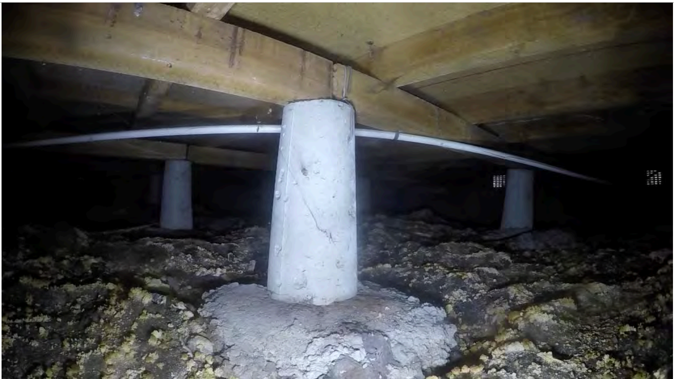
28: Pile with bearer join. There is significant yellow mold growing beneath this home.
