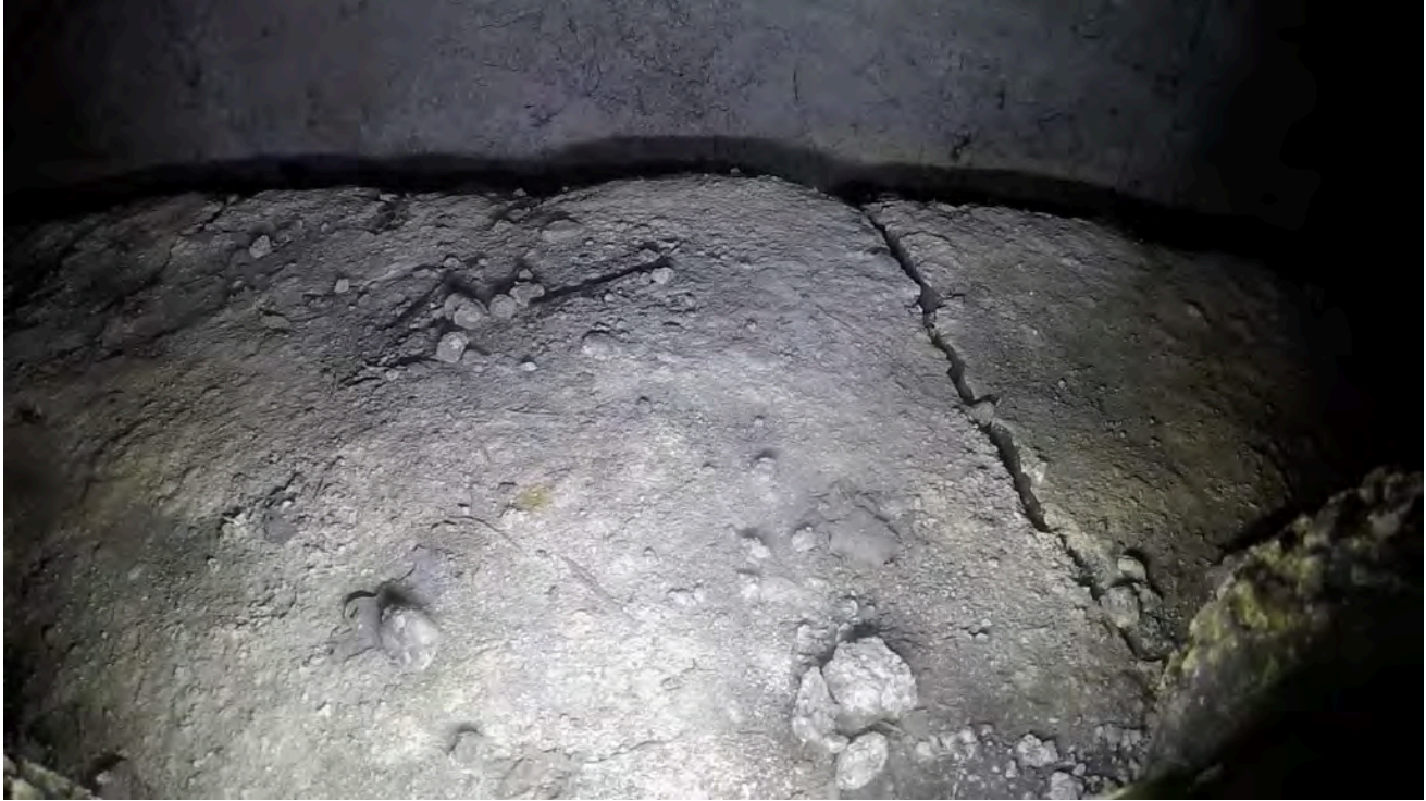
9: Large ground crack heading towards the foundation.
