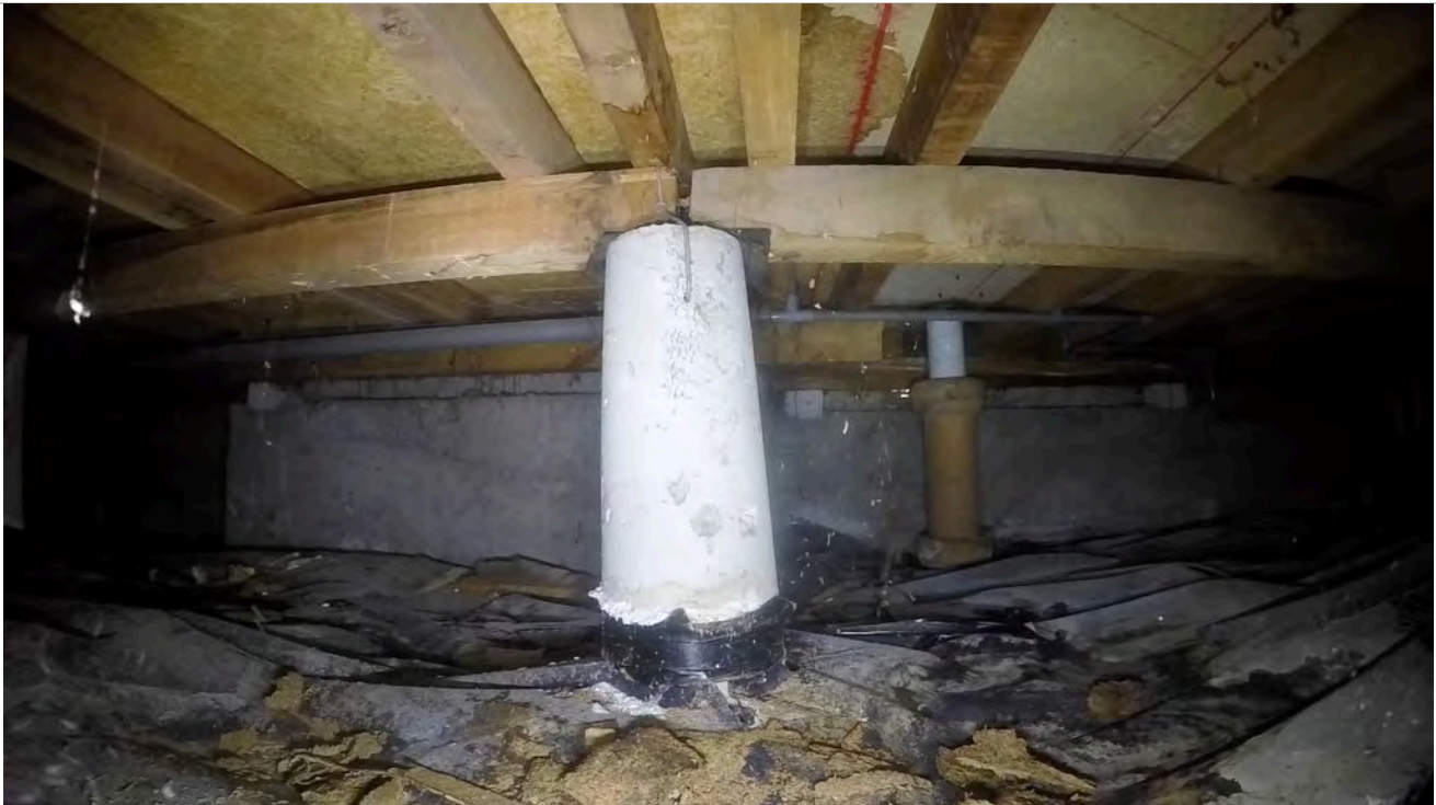
38: There are indications of an above floor water leak here and the timber is showing signs of water damage.
