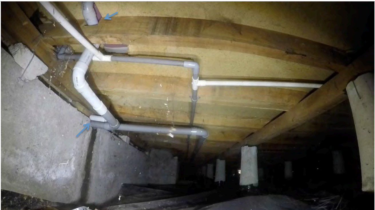
44: View of ring foundation with services. The joist has been notched by at least 40mm. There is evidence that the wastewater is flowing back into the foundation from the gully.
