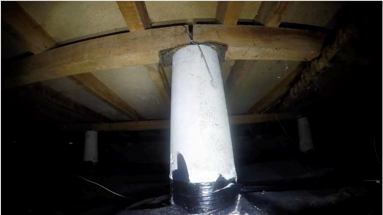
20: Pile with bearer join. The bearer join has pulled apart. This is most likely caused by timber shrinkage. The subfloors were generally constructed from wet timber, which reduces in size when dry.
