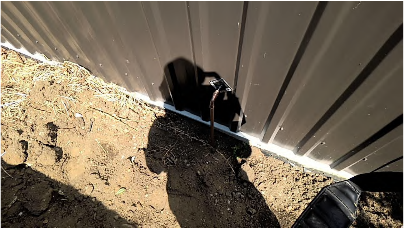
Cold water feed
