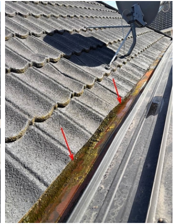
Roofing iron starting to rust. This should be treated. Above garage
