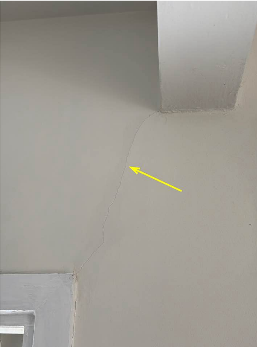
Example of cosmetic cracking noted.
