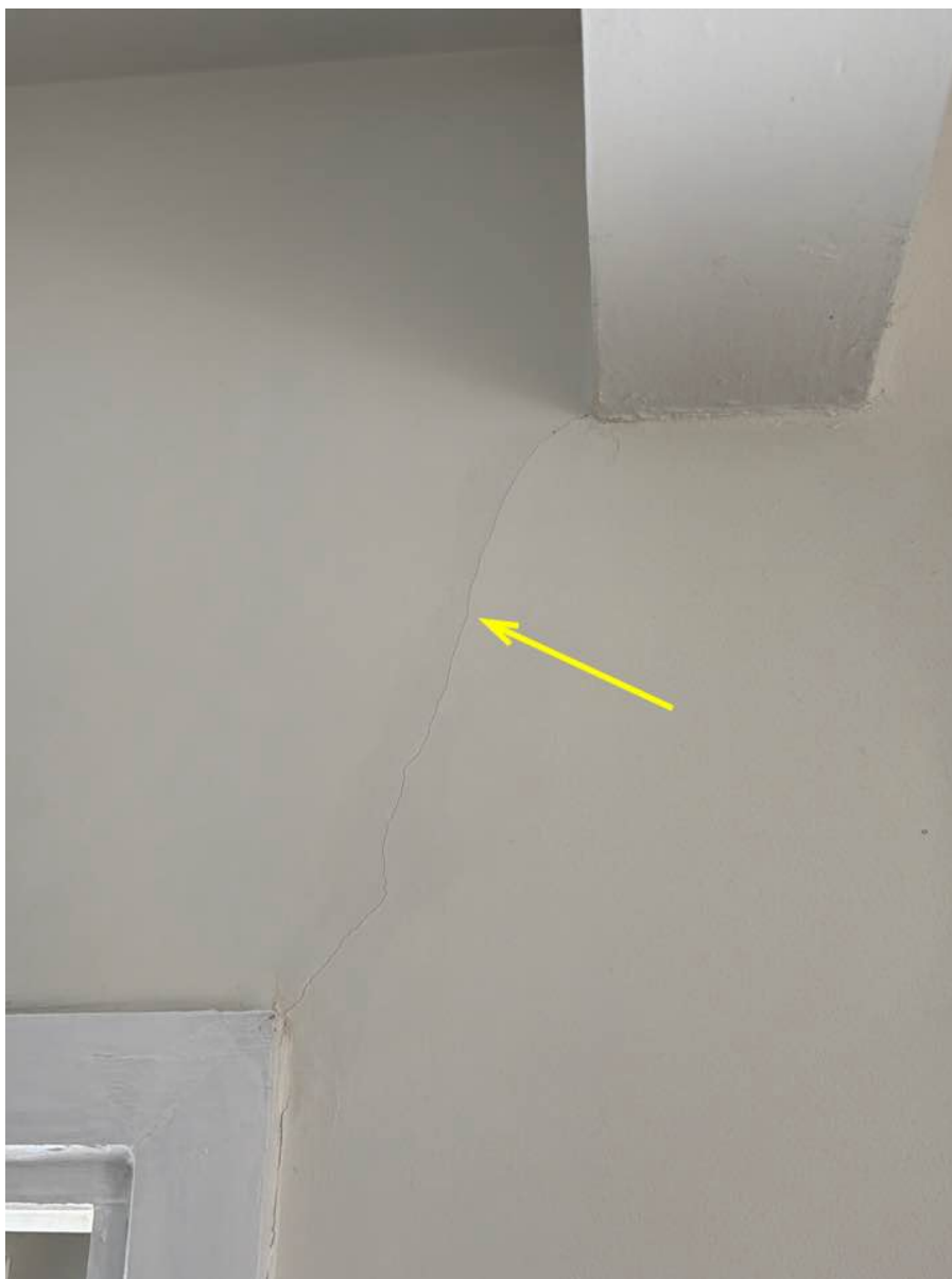
Example of cosmetic cracking noted.
