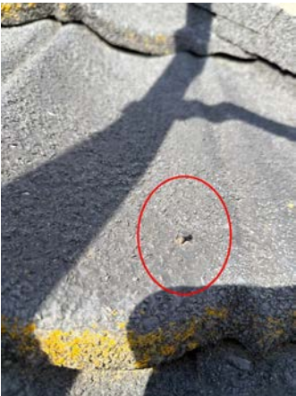
Example of popped roof cladding fixings.
