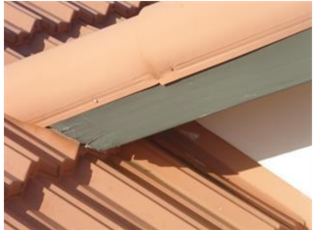
End grain deterioration
