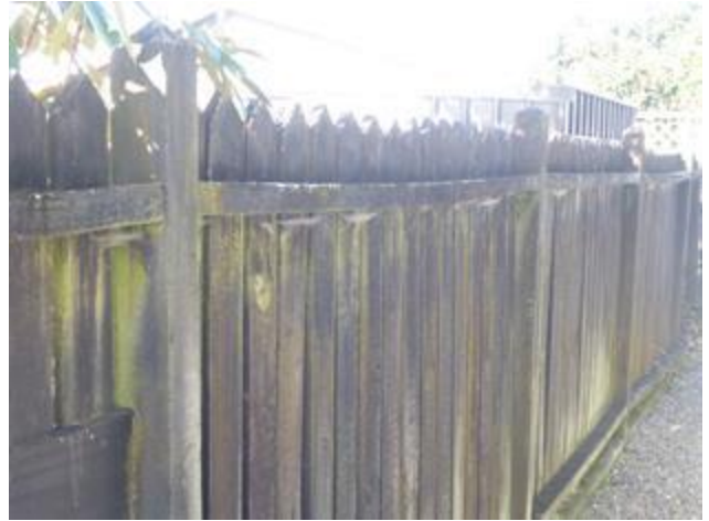
Post repair recommended
