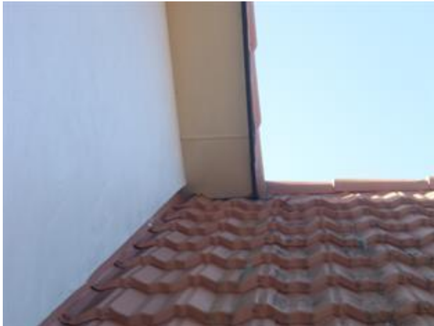
Fascia and soffit in contact
