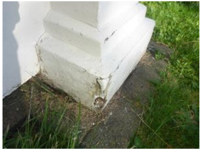
Impact damage front
