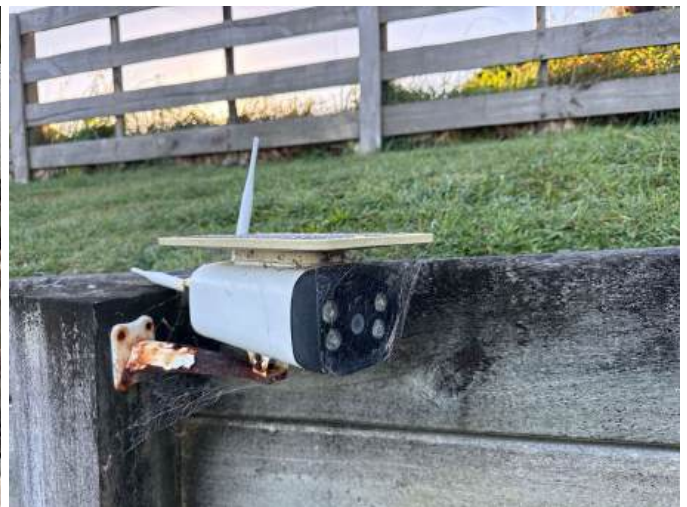
Security camera system installed. Untested.
