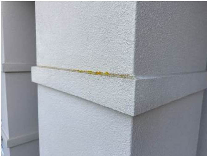
Lichen should be removed for the cladding surface to prevent the risk of premature deterioration
