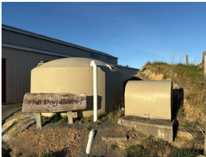
Fire fighting tank and generator installed by shed. The generator, water pumps and condition of the tanks were not checked as part of the inspection process.
