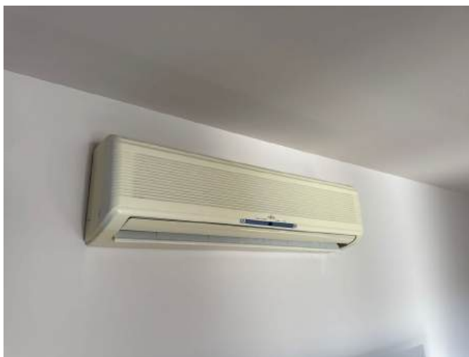
Heatpump installed. Untested.
