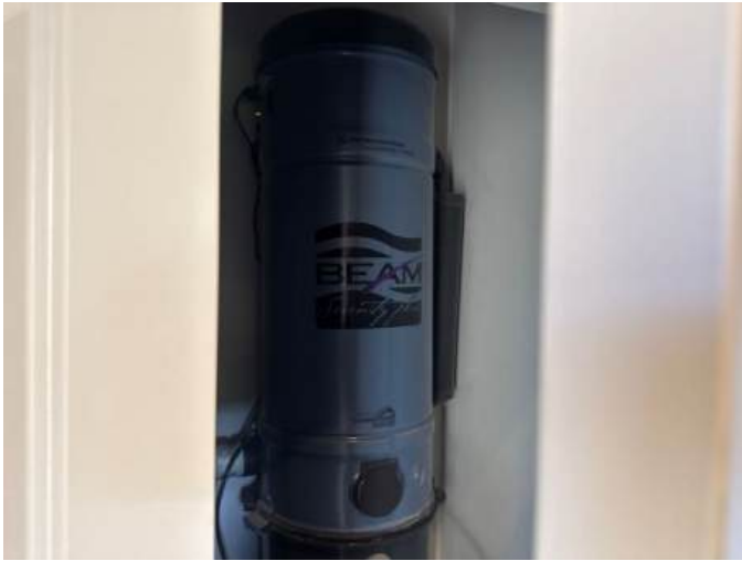
A central vacuum system is located inside the laundry cupboard. Untested.
