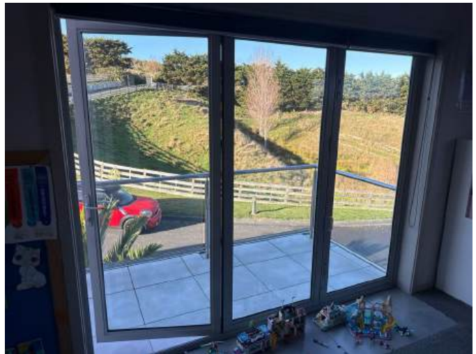
The bifold door is functioning
