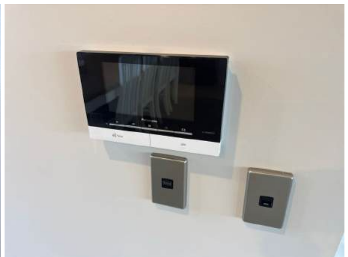
Intercom and gate control is located in the dining area.
