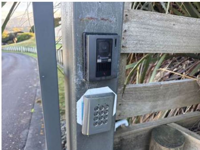
Intercom and camera to to the gate entrance
