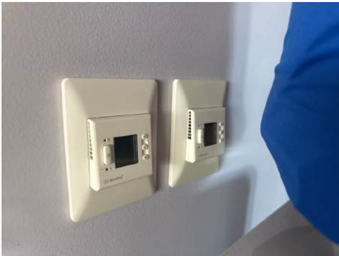
Control panels for the under tile heating are located in the kitchen and bathrooms
