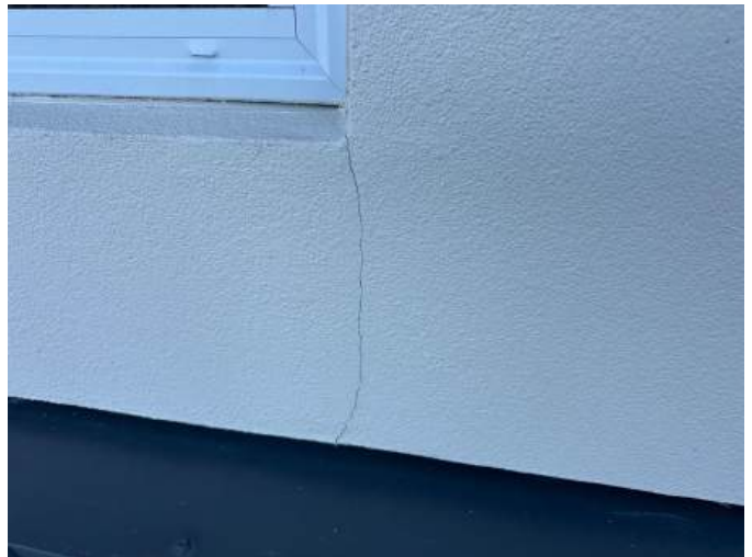
West/Southwest side above garage roof. Hairline cracking requires repair.
