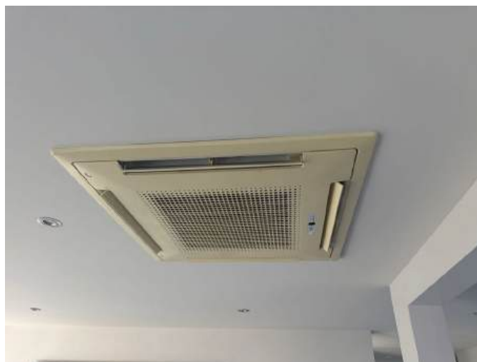
Ceiling Heatpump installed.
